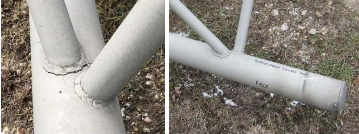
Figure 3: Partial fracture observed at second location within truss
