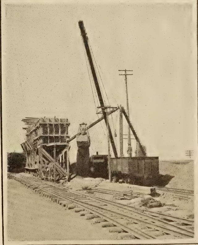
MACHINERY ON MINNESOTA FEDERAL-AID PROJECT NO. 31. TOP—STEEL STONE AND SAND BOXES AT MIXING PLANT. SUBGRADE AND FORMS READY TO RECEIVE CONCRETE SURFACING. BOTTOM—SAND AND STONE STORAGE BINS, CRANE AND CLAM SHELL BUCKET AT RAILROAD SIDING.
