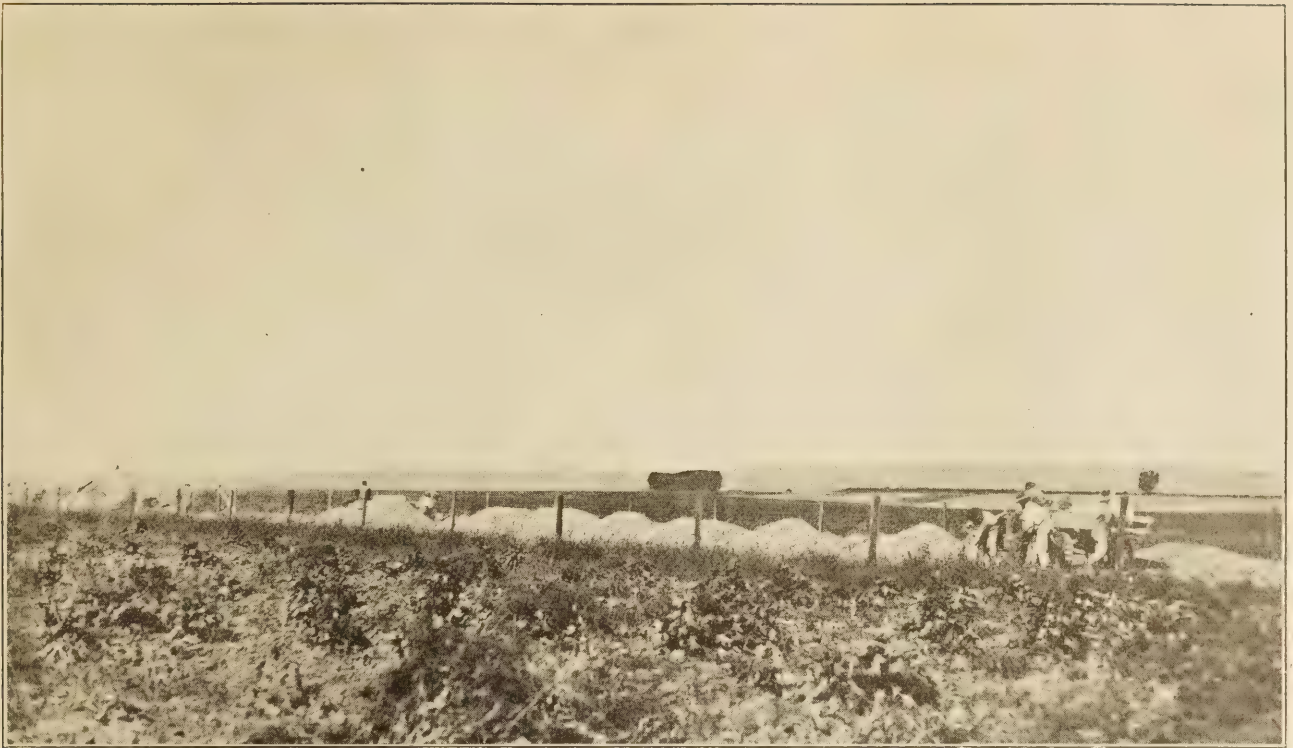
STOCK PILES, SHOWING LABORERS LOADING A TRUCK, ON A FEDERAL-AID PROJECT IN WYOMING.
