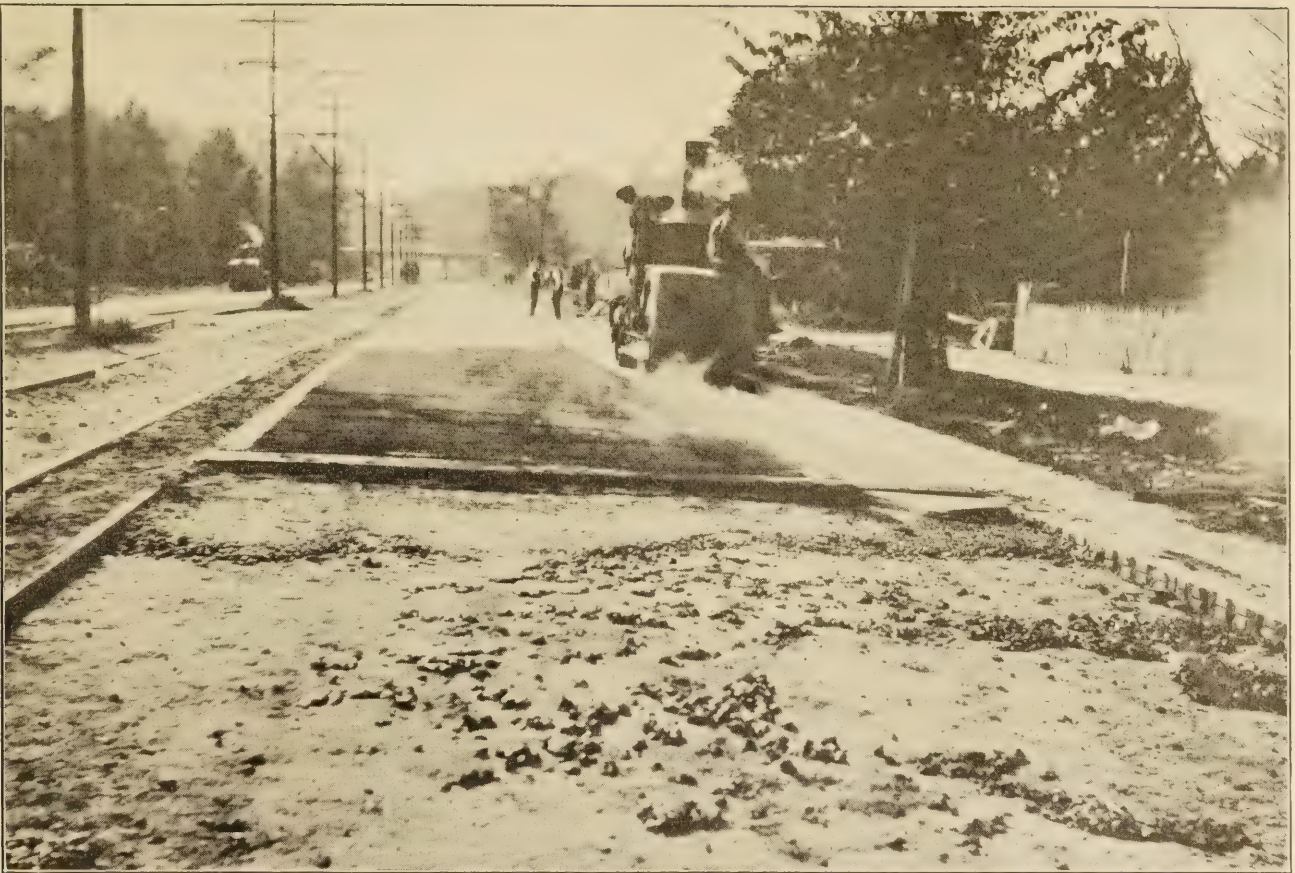
CONCRETE BASE, BINDER COURSE, AND ROLLING ASPHALT TOPPING, RHODE ISLAND AVENUE NE., WASHINGTON, D. C., OCTOBER, 1919.
