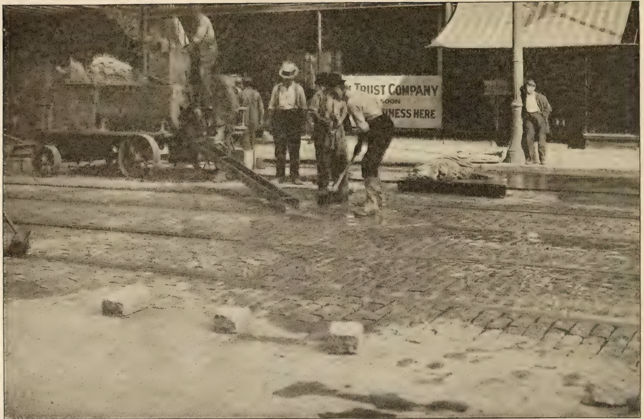
GROUT MIXED BY MACHINE TO PROPER CONSISTENCY TO FLOW READILY TO BOTTOM OF JOINTS.
