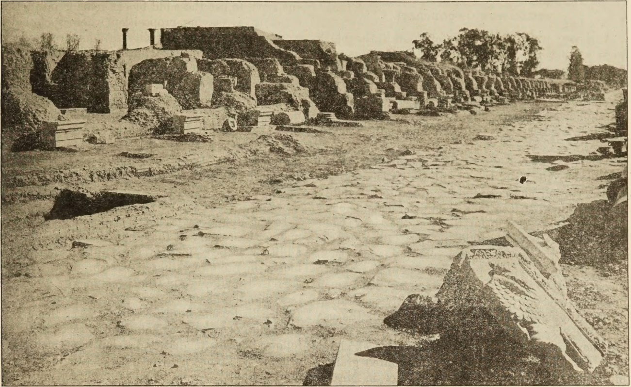
PORTION OF THE APPIAN WAY, DECAYED AND NEVER REPAIRED, THOUGH MAJOR PART OF HIGHWAY, NOW 2,000 YEARS OLD, IS IN GOOD CONDITION.
