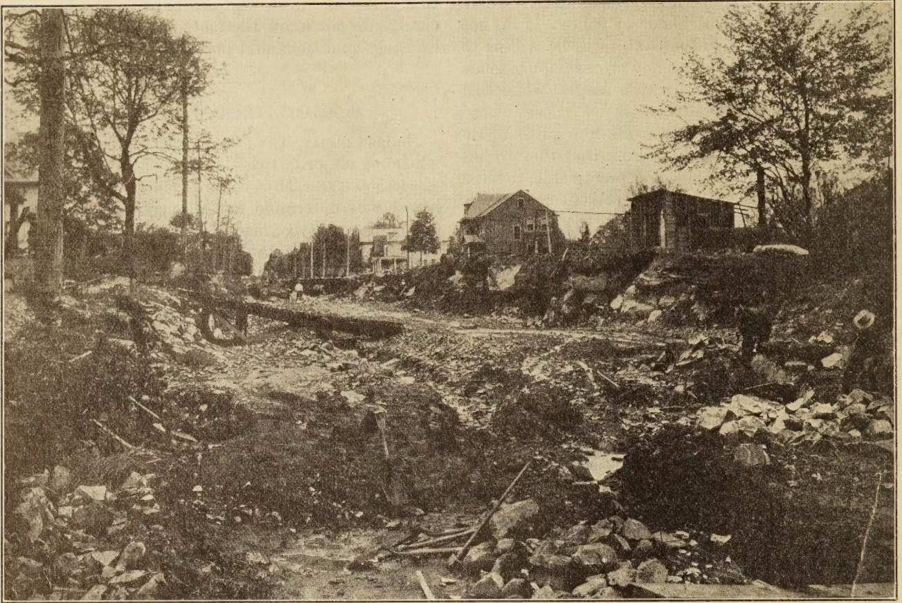
REDUCING AN 11 PER CENT GRADE TO 5 PER CENT ON DELAWARE PROJECT NO. 1A.
