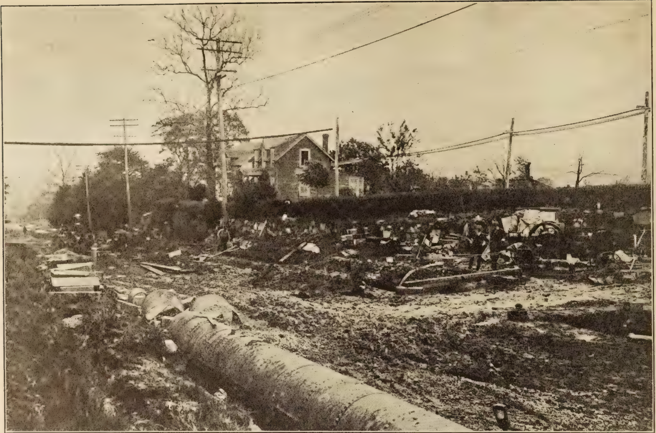
LOWERING TELEPHONE WIRE CONDUITS ON DELAWARE FEDERAL AID PROJECT NO. 1. NOTE THE TEMPORARY CABLE ON THE RIGHT.
