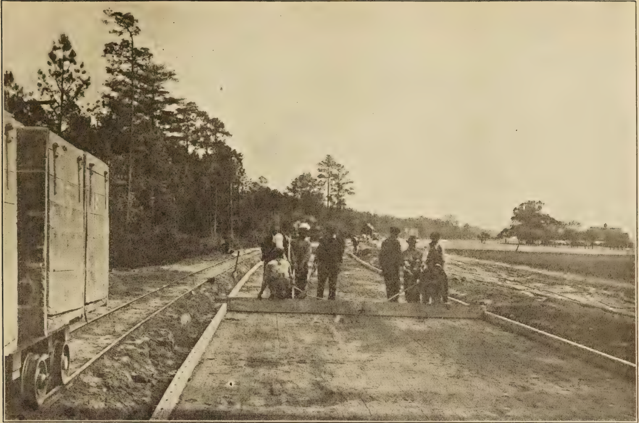
FINISHING THE SUBGRADE ON DELAWARE PROJECT NO. 4. NO MATERIALS LOST AND THE SUBGRADE UNIFORM.
