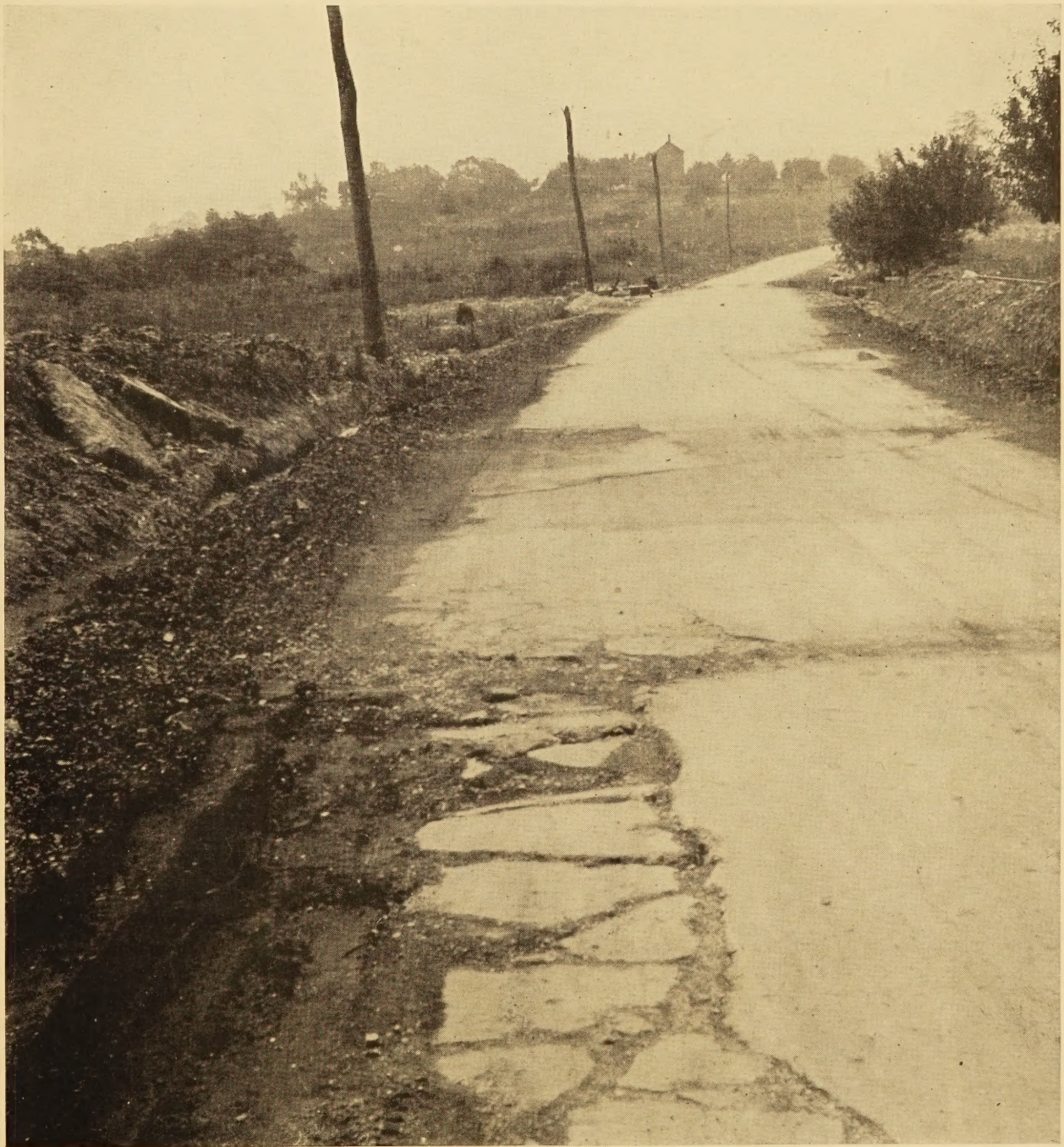
CONCRETE FAILURE DUE TO THE COMBINATION OF HEAVY LOADS AND WET SUBGRADE
