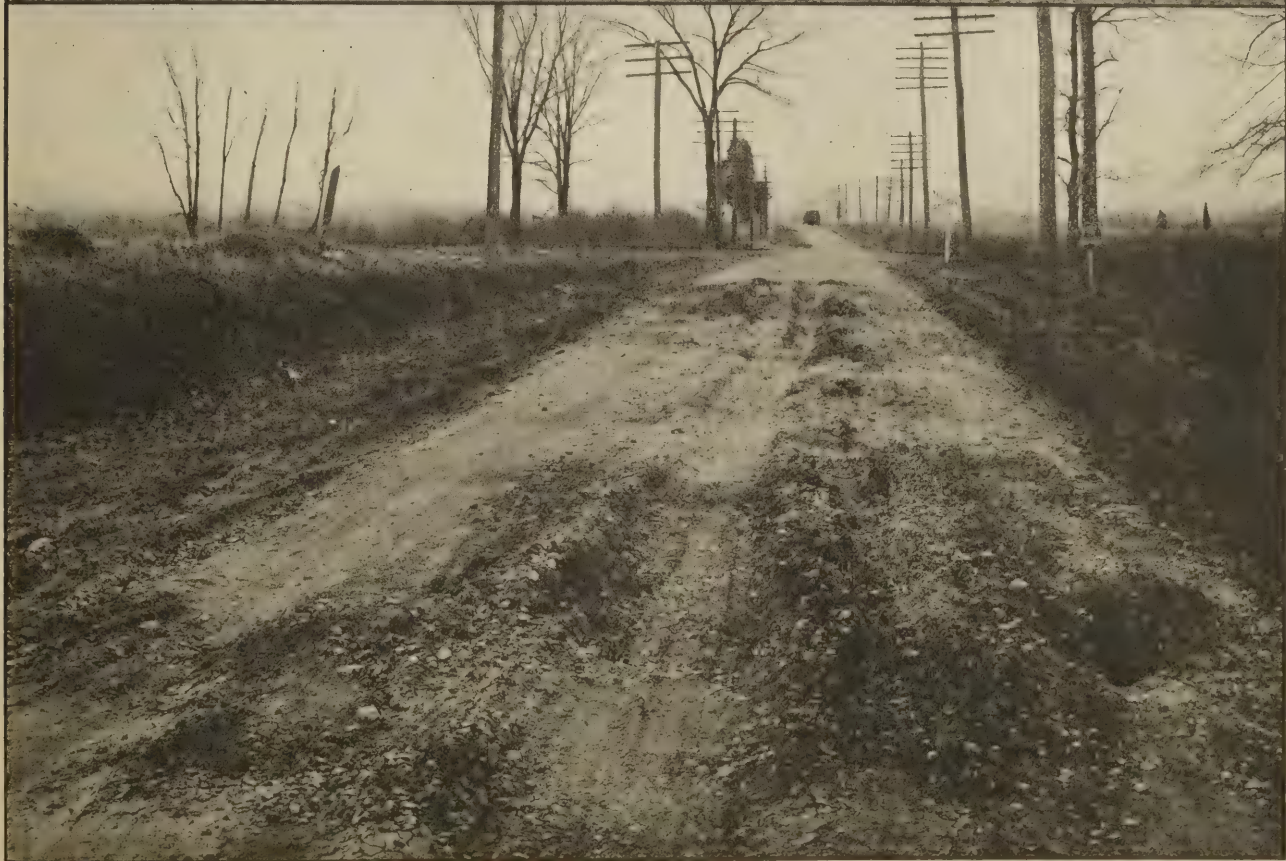
VIEWS OF TWO SECTIONS OF THE WASHINGTON-BALTIMORE BOULEVARD IN THE VICINITY OF SAVAGE, MD. THEY WERE CONSTRUCTED IN 1912, COST $12,000 A MILE, ARE OF MACADAM ON A CLAY SUBGRADE, 14 FEET WIDE, 8 INCHES THICK, WITH 5-FOOT SHOULDERS, AND WELL DRAINED. THEY STOOD UP WITH ORDINARY MAINTENANCE UNTIL THIS SPRING.
