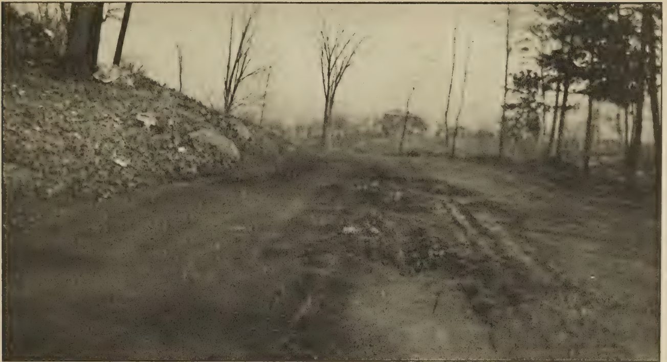
NEAR SUDBURY, MASS. WATER-BOUND MACADAM 6 INCHES THICK, BLANKET COAT ONE-HALF GALLON OF 90 PER CENT OIL IN 1910 AND 1911; ONE-HALF GALLON TAR IN 1909. ROAD BROKEN UP UNDER TRAFFIC, REPAIRED WITH ROAD SCRAPER BEFORE PHOTOGRAPH WAS TAKEN.
