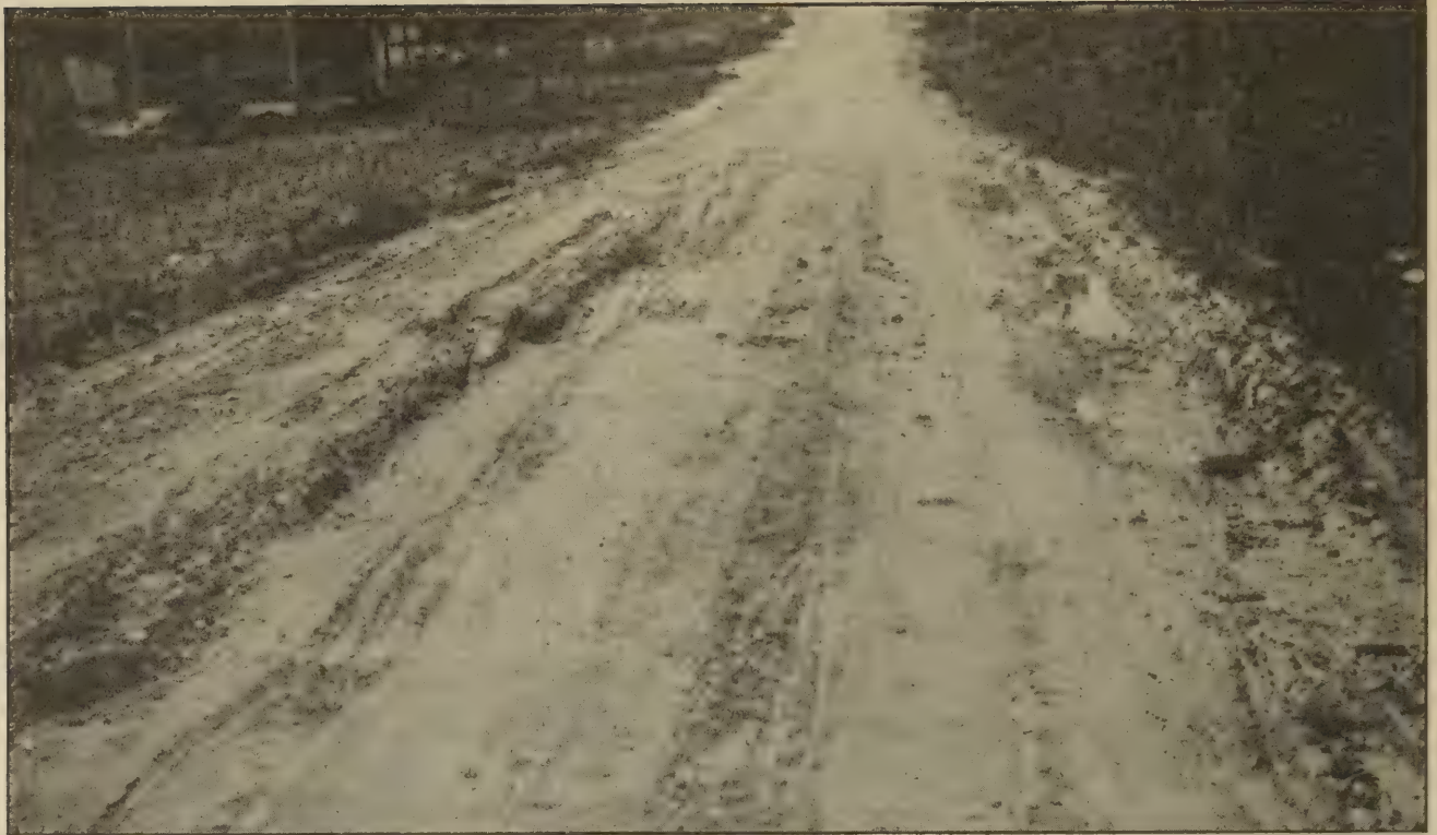
ON THE BELAIR ROAD AT CHURCHVILLE, MD. THIS ROAD, 14 FEET WIDE, 8 INCHES THICK, MACADAM, CLAY SUBGRADE, WAS CONSTRUCTED IN 1913 AT A COST OF $12,000 A MILE. IT IS WELL DRAINED AND WAS IN GOOD CONDITION PRIOR TO THE SPRING OF THIS YEAR, WHEN THIS PHOTOGRAPH WAS TAKEN.
