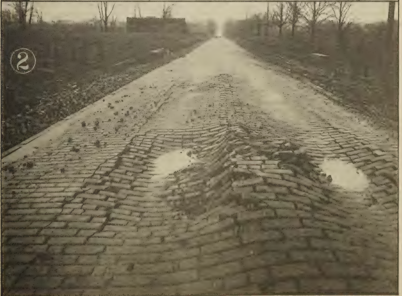
BRICK ON 4 INCHES OF CONCRETE ON THE CLEVELAND-AKRON ROAD NEAR ADSON, OHIO. AT TOP; PAVEMENT STILL IN GOOD CONDITION. BOTTOM: NEAR TWINSBURGH, BASE HAS FAILED, THOUGH BRICK ON THE TOP ARE STILL IN GOOD CONDITION EXCEPT WHERE DAMAGED BY FAILURE OF THE BASE.
