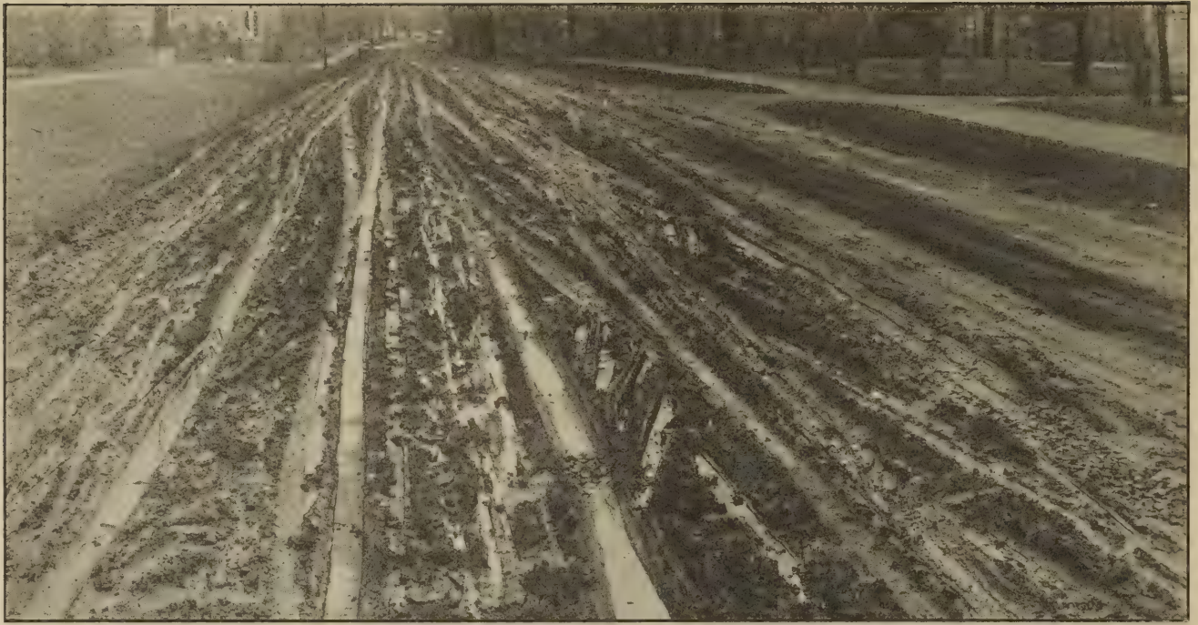
SECTION OF THE LENOX, MASS. STATE HIGHWAY. TRAP 16 FEET BY 6 INCHES BY 4 INCHES. RESURFACED WITH TRAP, 10 TONS TO 100 FEET IN 1908. PATCHED IN 1911 STANDARD A ONE-HALF GALLON PER SQUARE YARD, ONE-FOURTH GALLON PER SQUARE YARD LIGHT OIL IN 1914 AND ONE-FIFTH GALLON IN 1916.
