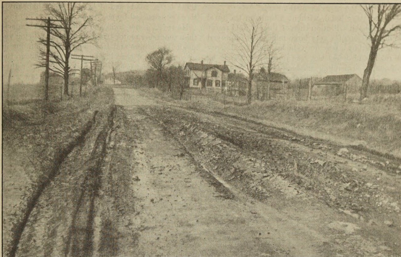
MOVING VANS, PRODUCE, AND FREIGHT TRUCKS PUT THIS MACADAM ROAD BETWEEN VICTOR AND MENDON, N. Y., INTO THE CONDITION SHOWN. ESTIMATED COST OF REPAIR IS $20,000 PER MILE.
