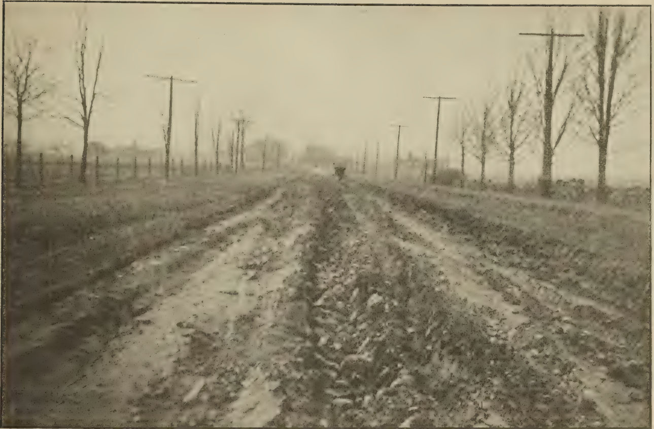
THIRTY 7-TON UNITS PER DAY BROKE UP THIS BITUMINOUS MACADAM ROAD IN LIVINGSTON COUNTY, N. Y. IT IS ESTIMATED THAT REPAIRS AT PRESENT PRICES WILL COST $32,000 PER MILE FOR PROBABLY 14 MILES.
