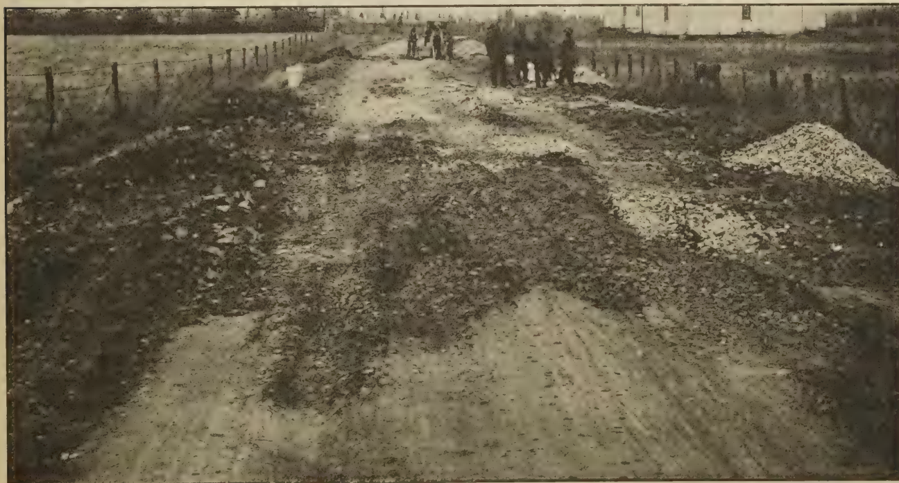
AT TOP—FAILED SECTIONS ON CONCRETE ROAD BETWEEN ABERDEEN AND ELKTON, MD. AT BOTTOM—THE WASHINGTON-BALTIMORE BOULEVARD AT MUIRKIRK MD., COST $15,000 A MILE TO BUILD IN 1913. IT IS 14-FOOT MACADAM, 8 INCHES THICK, CLAY SUBGRADE, 5-FOOT SHOULDERS, AND WELL DRAINED. LIKE OTHER ROADS, IT WAS IN GOOD CONDITION UNTIL THIS SPRING.
