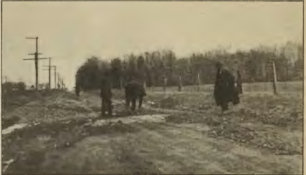
ON THE MAIN ROAD, PHILADELPHIA TO NEW YORK, NEAR WINDSOR, N. J. WATERBOUND MACADAM, BITUMINOUS DRESSING, BUILT IN 1915. GOOD IN FALL OF 1917 AND CARRYING 172 HEAVY UNITS A DAY.
