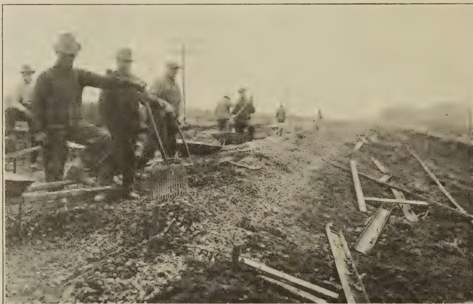
Showing materials for concrete distributed on road bed and manner of handling same to mixer. Iowa Federal Aid Project.
