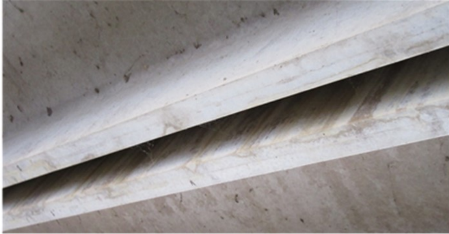
Figure 3.6 Example of efflorescence on Bridge B (Credit: Brian Kidd)
