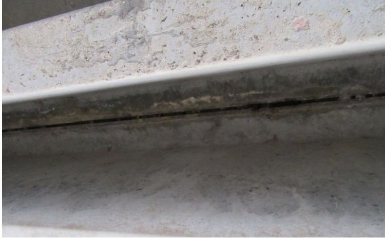
Figure 3.3 Efflorescence and erosion between G7 and G6 on Bridge A (Credit: Brian Kidd)
