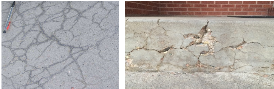
Figure 2.3 ASR damage in Wyoming a) map cracking at Federal Street in Riverton and b) pop-outs combined with map cracking in Cheyenne
