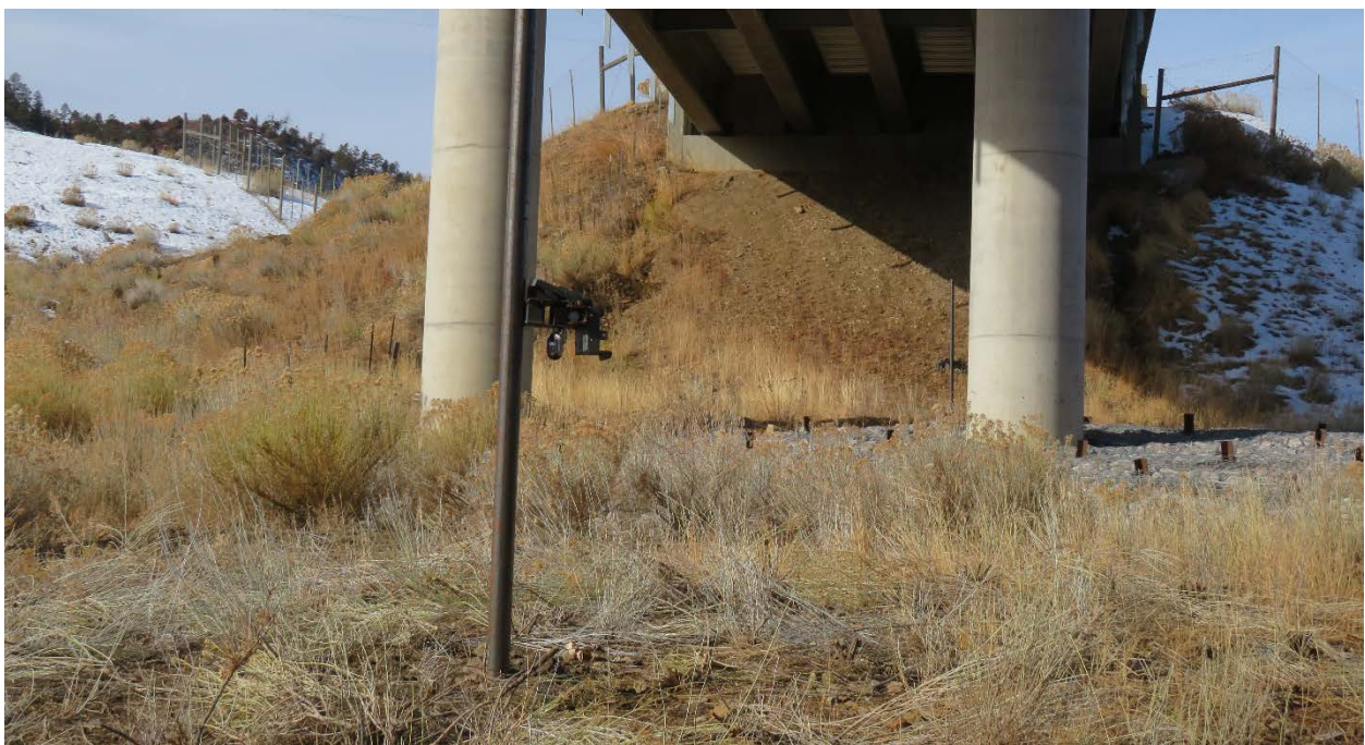
Figure 18. Pole B installation, looking west (pole A in the background to the left of the right-most pier).
