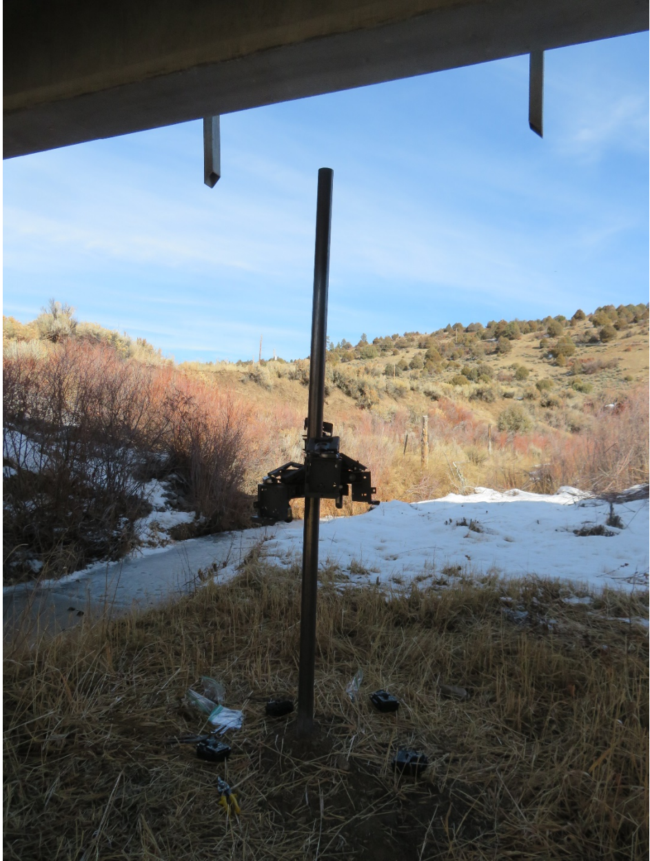
Figure 13. Pole installation at bridge #9387 looking north with Amargo Creek visible to the left of the pole.
