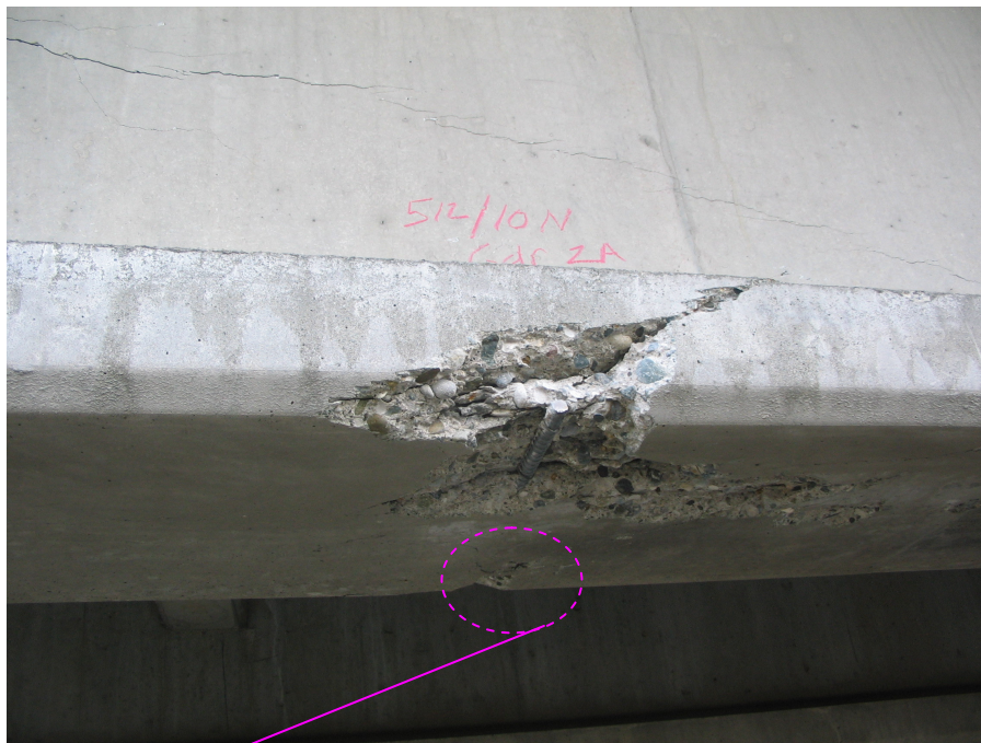
(c) Comparison with the real scenario (as shown in the photo, the impact loading position is a little bit away from the intermediate diaphragm, and a small area of the tensile failure developed on the back face of the girder flange, the same as showed in the simulation plots of (a) and (b))
