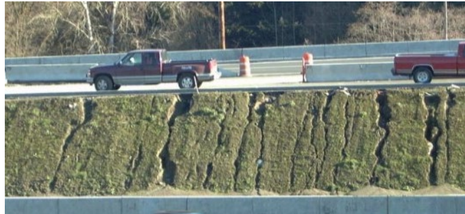
Figure 1. Excessive rilling and erosion near a roadway construction site.
