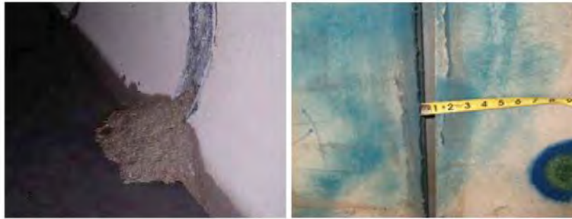
RCP Examples With Joint Separation, Missing Seal and Backfill Loss
