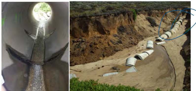
78 in. RCP with Misalignment
