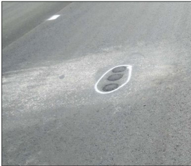
Photograph 16 - Obvious Defect (Improperly Repaired Core Holes)
