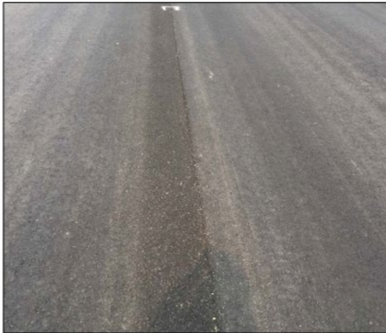
Photograph 14 - Improperly Matching Joint (View 1)
