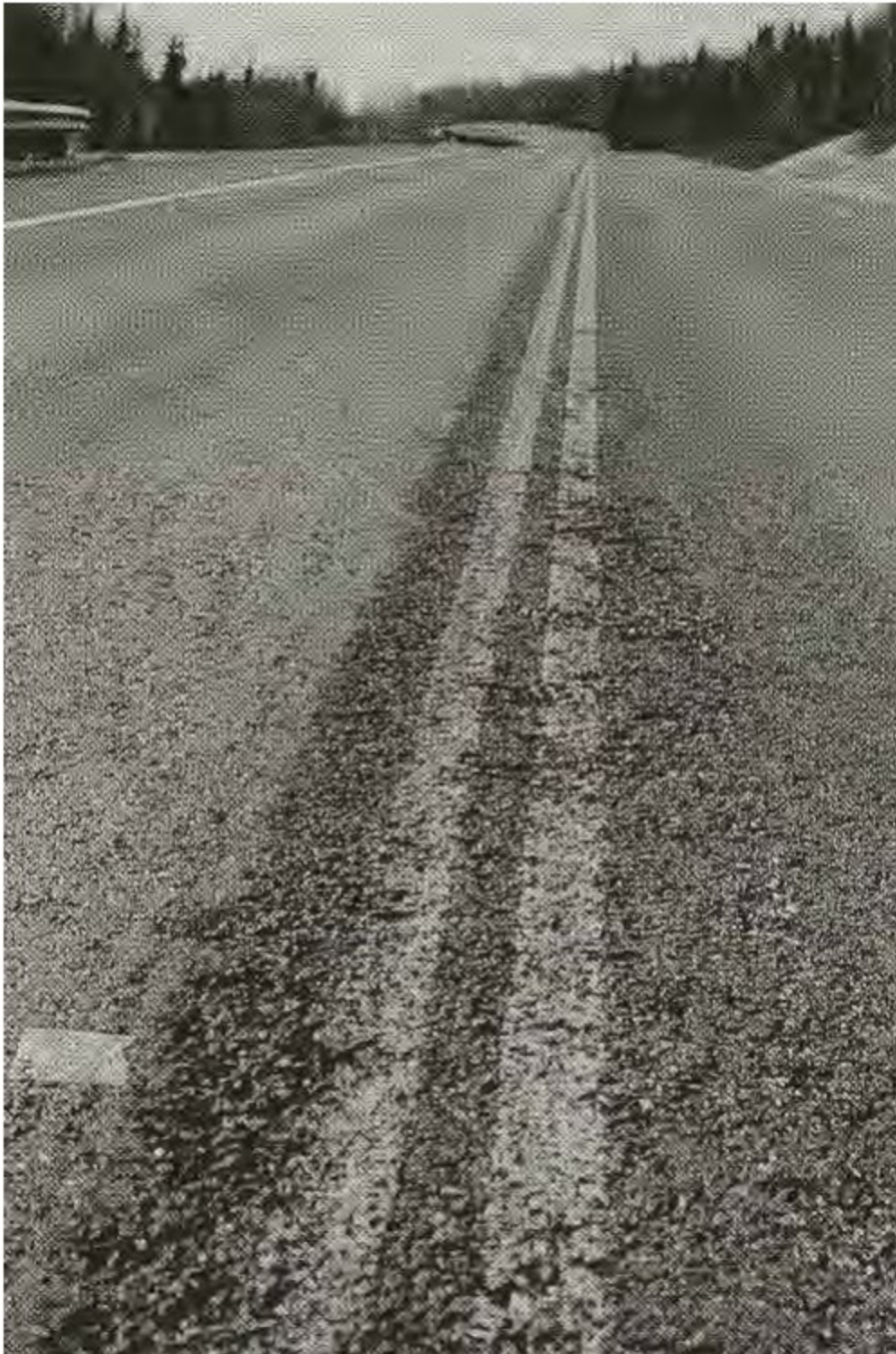
Figure 6-14 Segregation Visible in the Finished Mat
