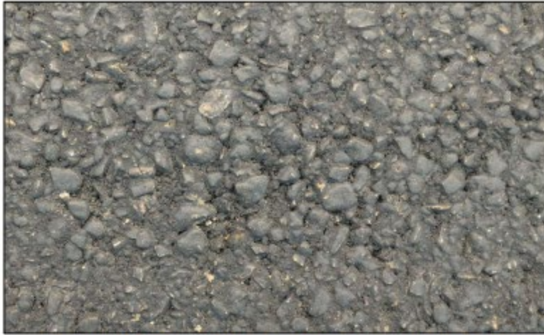
Photograph 9 - Moderate Segregation (bordering on Severe) (Close-Up)
