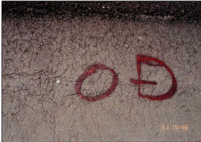
Photograph 17 - Obvious Defect (Hairline Cracking)
