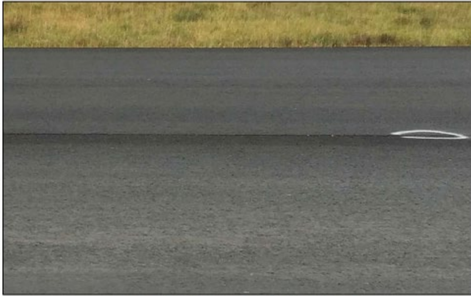
Photograph 15 - Improperly Matching Joint (View 2)
