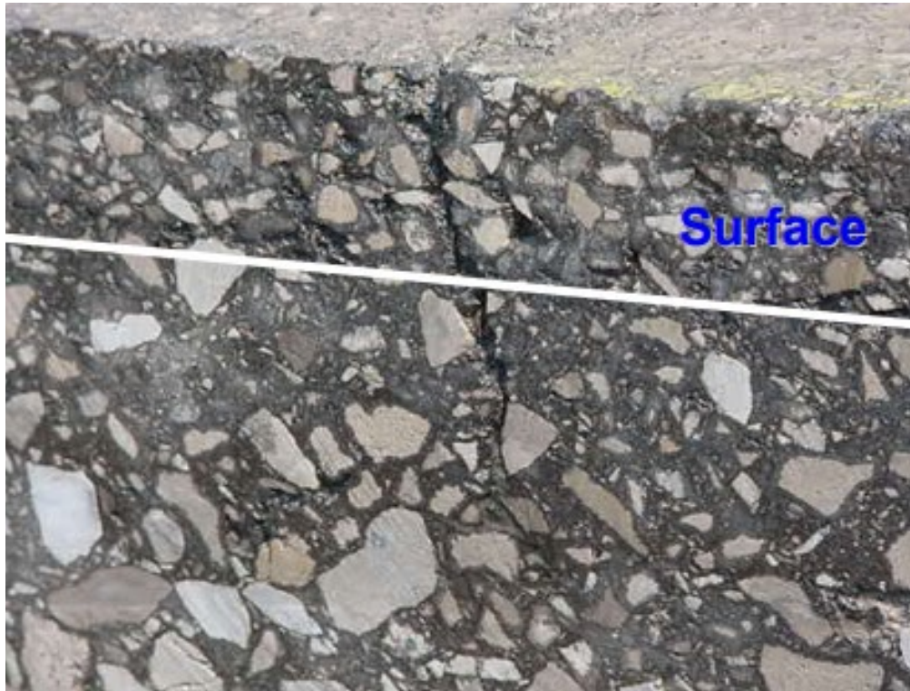
Figure 2. Close-up of longitudinal surface crack in DEL-23 SHRP Test Road, with white line added indicating where segregation was observed in the specimen [Sargand et al., 2006].
