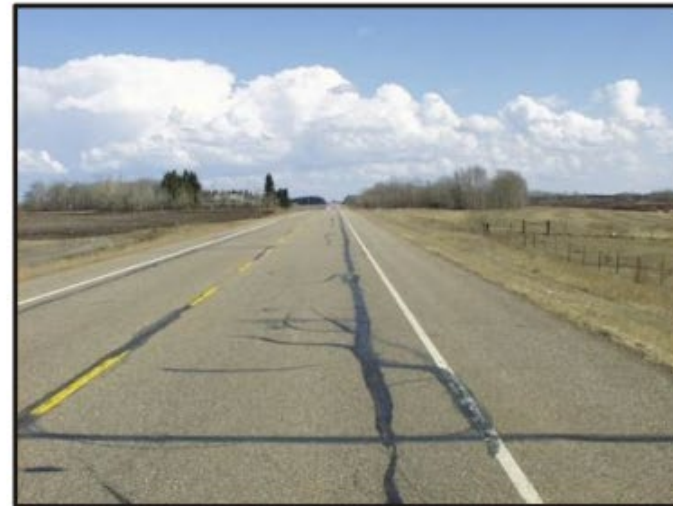
Centre-of-Paver Crack Located in Outer Wheel path
