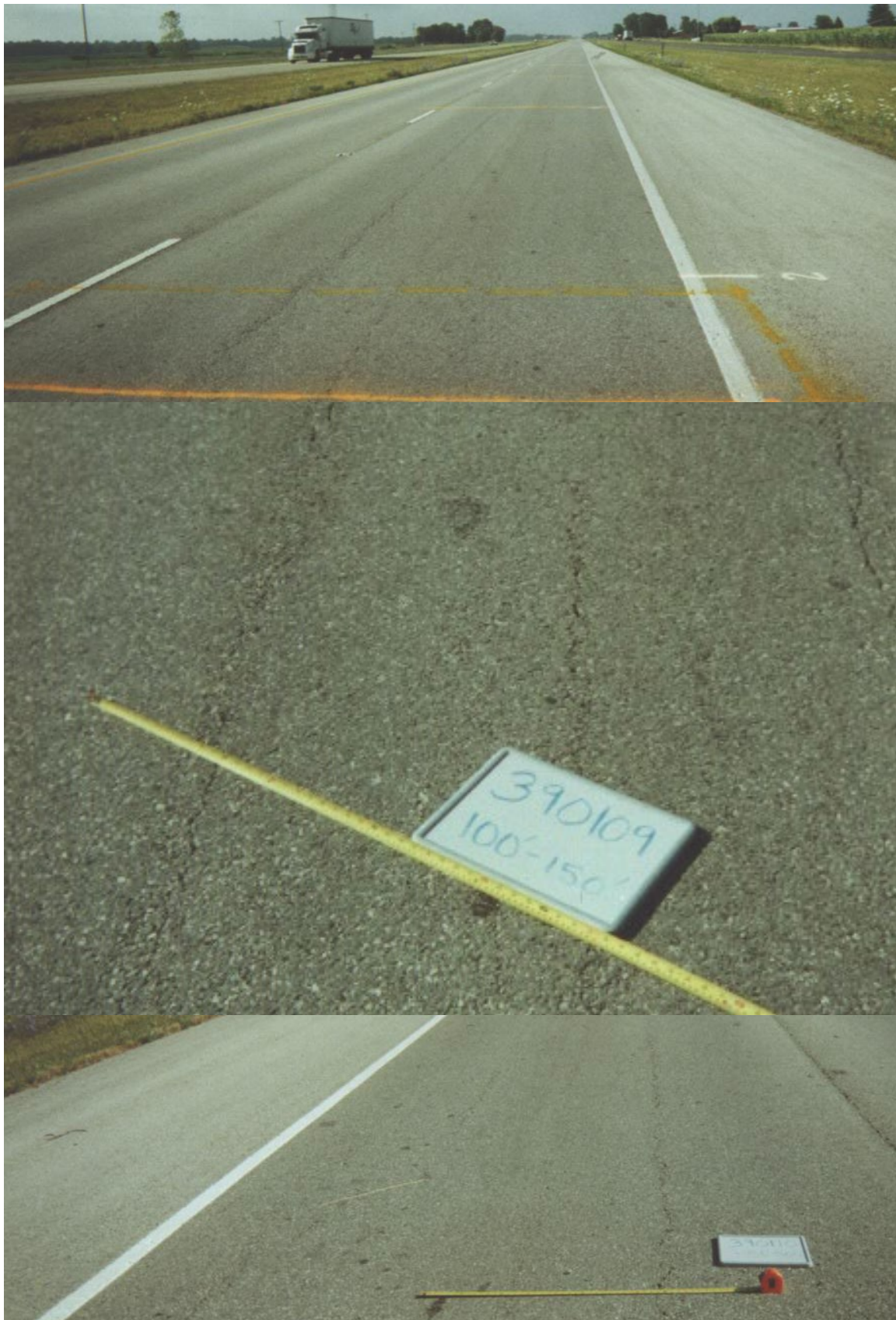
Figure 1. Longitudinal surface cracks in DEL-23 SHRP Test Road sections 390108, 390109, and 390110 [Sargand et al., 2006].
