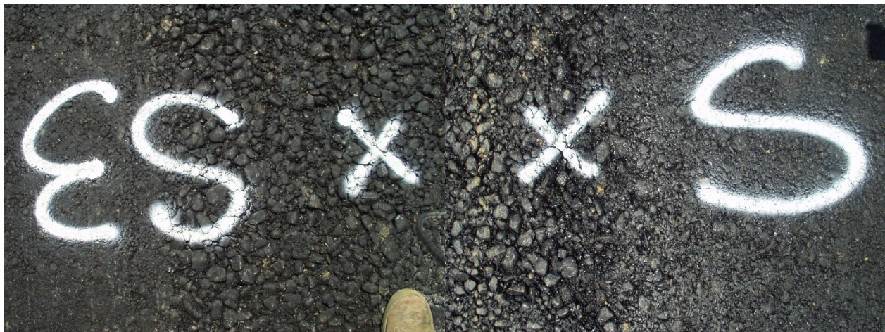
Figure 3. Segregation observed in asphalt base course on WAY 30 [Sargand, 2006, slides 30-31].
