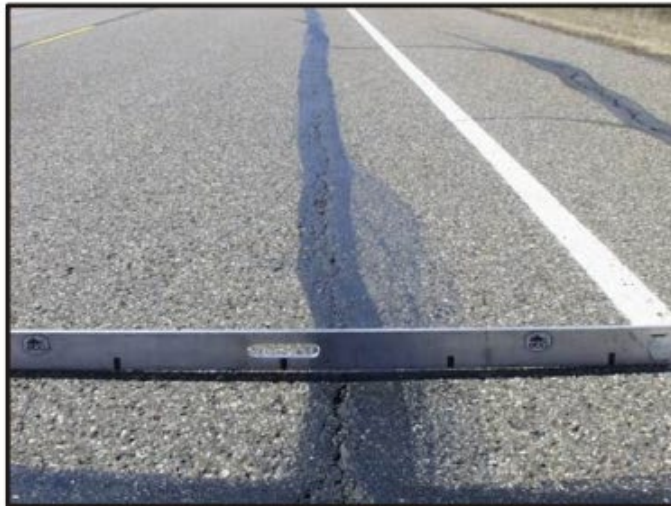
Moderate Severity Centre-of-Paver Crack
