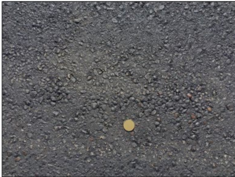
Photograph 4 - Slight Segregation (Close up)
