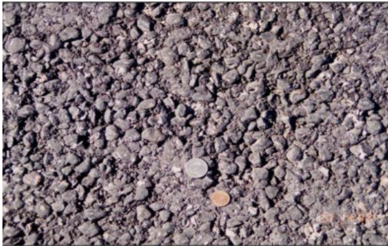
Photograph 12 - Severe Segregation (Close-Up)
