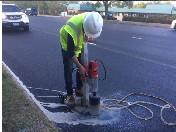
Figure A.11 Pictures Taken during Construction of Test Sections in the City of Kettering (Project No. 5).
