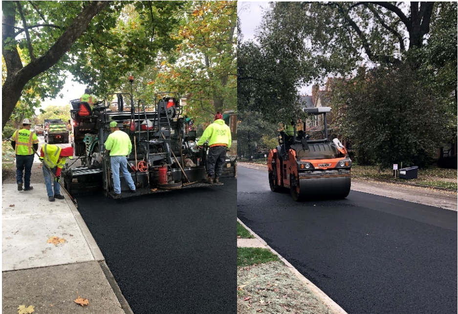
Figure A.8 Pictures Taken during Construction of Test Sections in Columbus Project 2.
