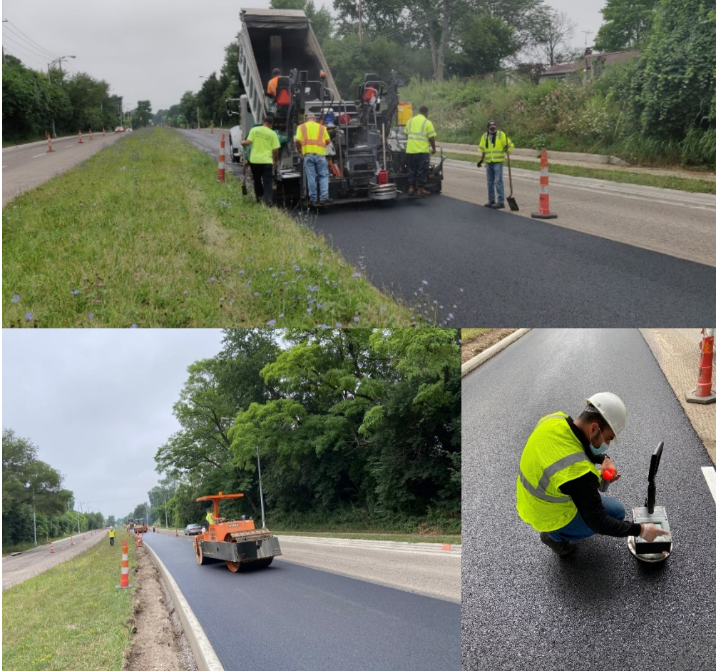
Figure A.7 Pictures Taken during Construction of Test Sections in the Columbus Project 1.
