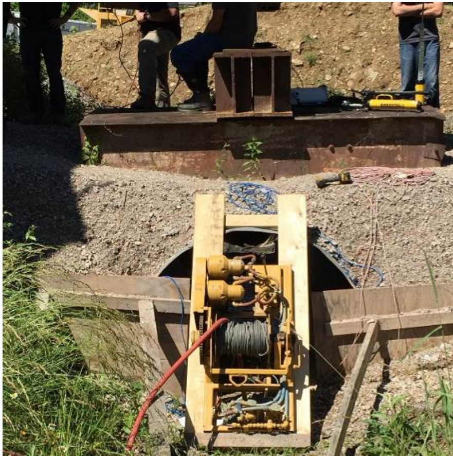
Figure 28. Winch placed at exit of the pipe to pull the re-rounder through.
