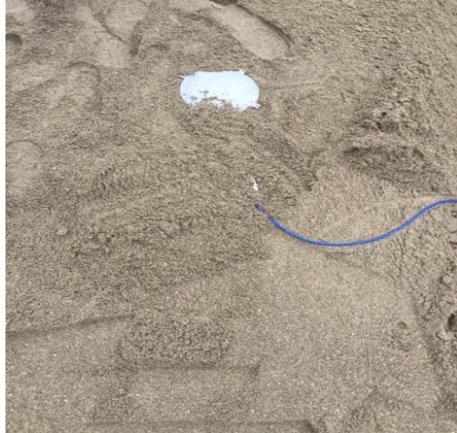
Figure 23. GEOKON pressure cell above crown of the pipe.
