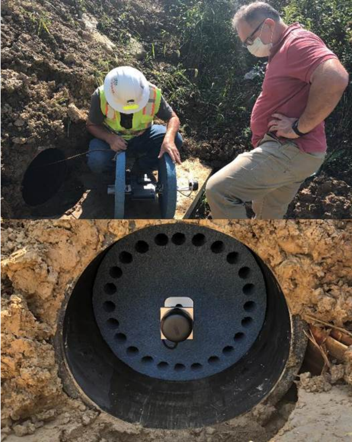
Figure 50. LiDAR profiler being used on Test Pipe 4. Top: Profiler being prepared by graduate student for insertion; Bottom: Profiler inside pipe.
