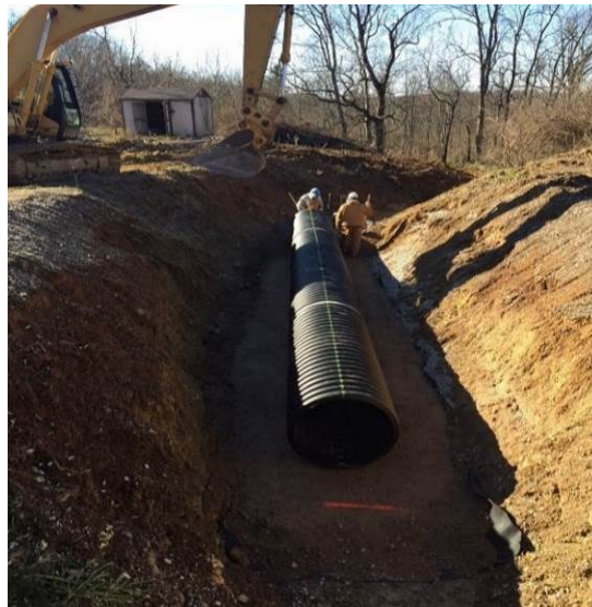
Figure 14. Corrugated HDPE pipe fabricated from three sections placed on a 6-in (0.15 m) bed of ODOT. C&MS Item 304.
