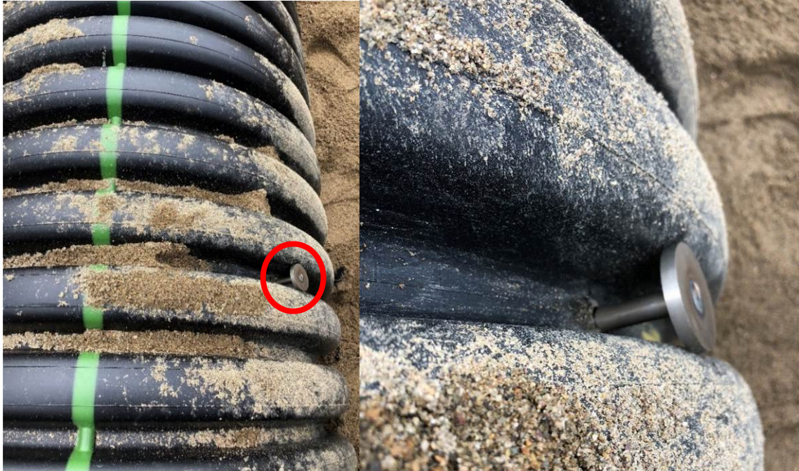
Figure 35. Left: The circled apparatus was installed at the shoulder of the pipe to measure soil resistance before and after re-rounding; Right: A closer view of the device.
