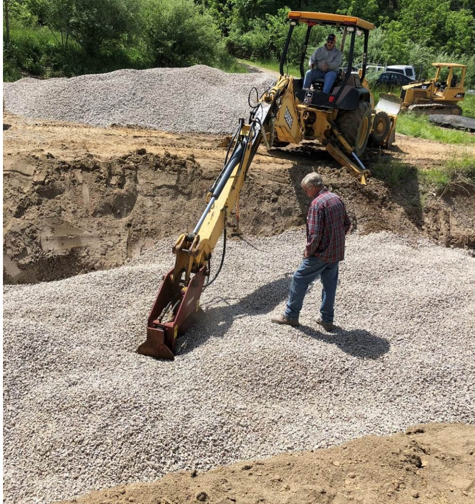
Figure 39. Compaction of the Structural Backfill Type 3 over Test Pipe 3 using a hydraulic plate compactor.
