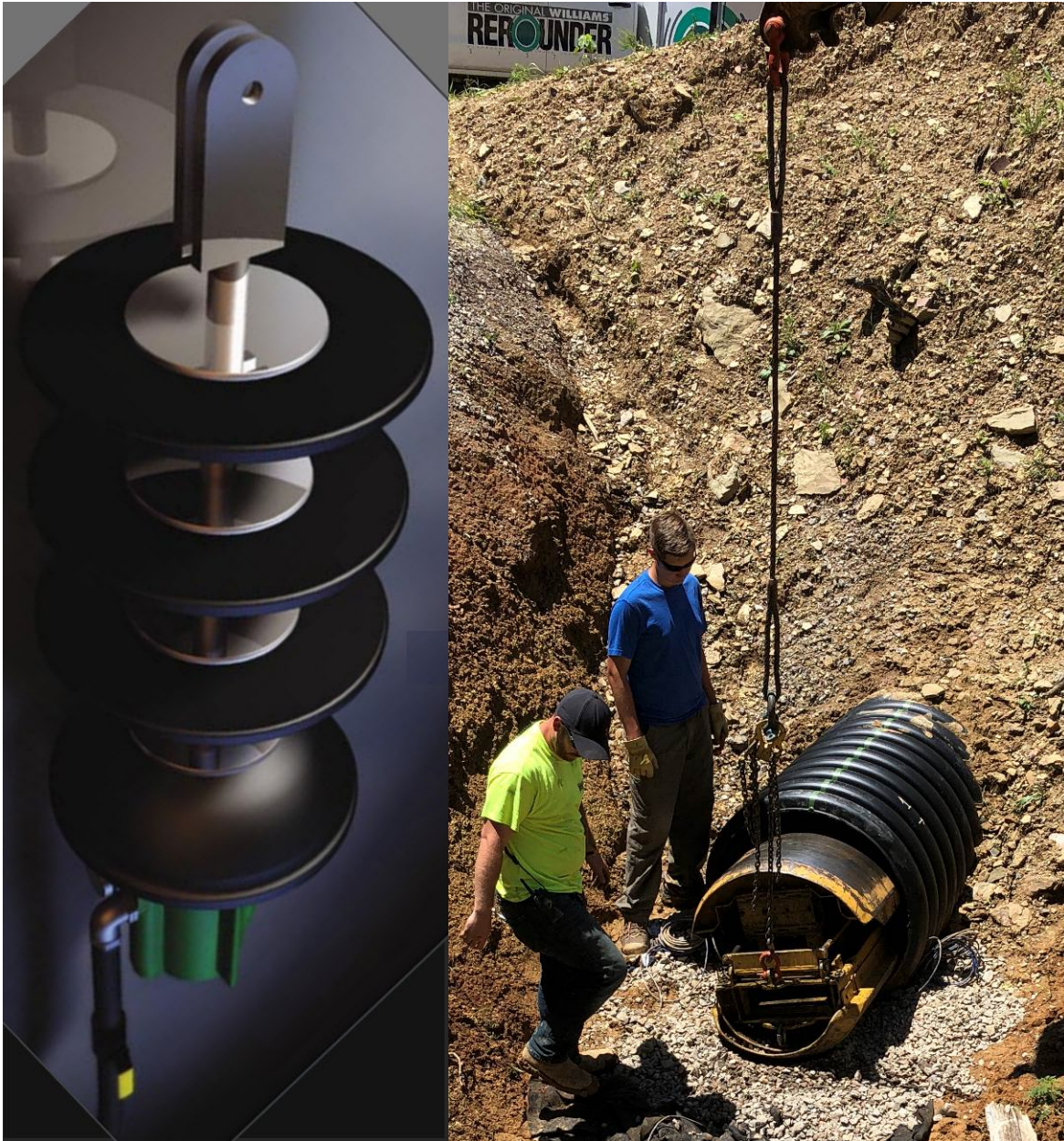
Figure 13. Re rounding devices: Hurco Re-rounder™ (left, adapted from Hurco brochure [Hurco, 2005]) and Williams re-rounding device in 36 in (0.9 m) diameter pipe (right).
