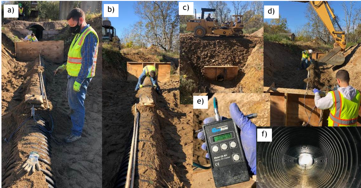
Figure 51. Views of installation of Test Pipe 5 on October 22, 2020: a) Testing accelerometer; b) Levelling backfill above crown in preparation for placing accelerometer; c) Placement of second (higher) accelerometer; e) Checking pressure cell readout; f) view inside pipe.
