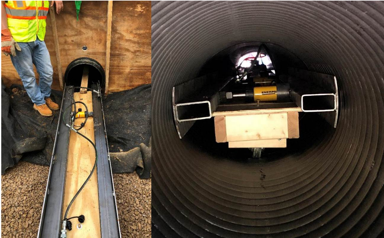
Figure 47. The pipe deflector was used to deform Test Pipe 4 during installation. Left: Deflector being inserted into pipe. Right: Deflector in operation.
