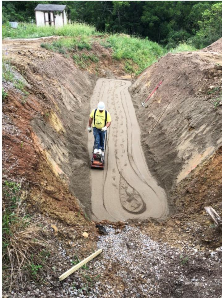
Figure 29. Compacting the 6-in (150 mm) bedding layer of ODOT Type 2 backfill sand before placing Pipe 2.
