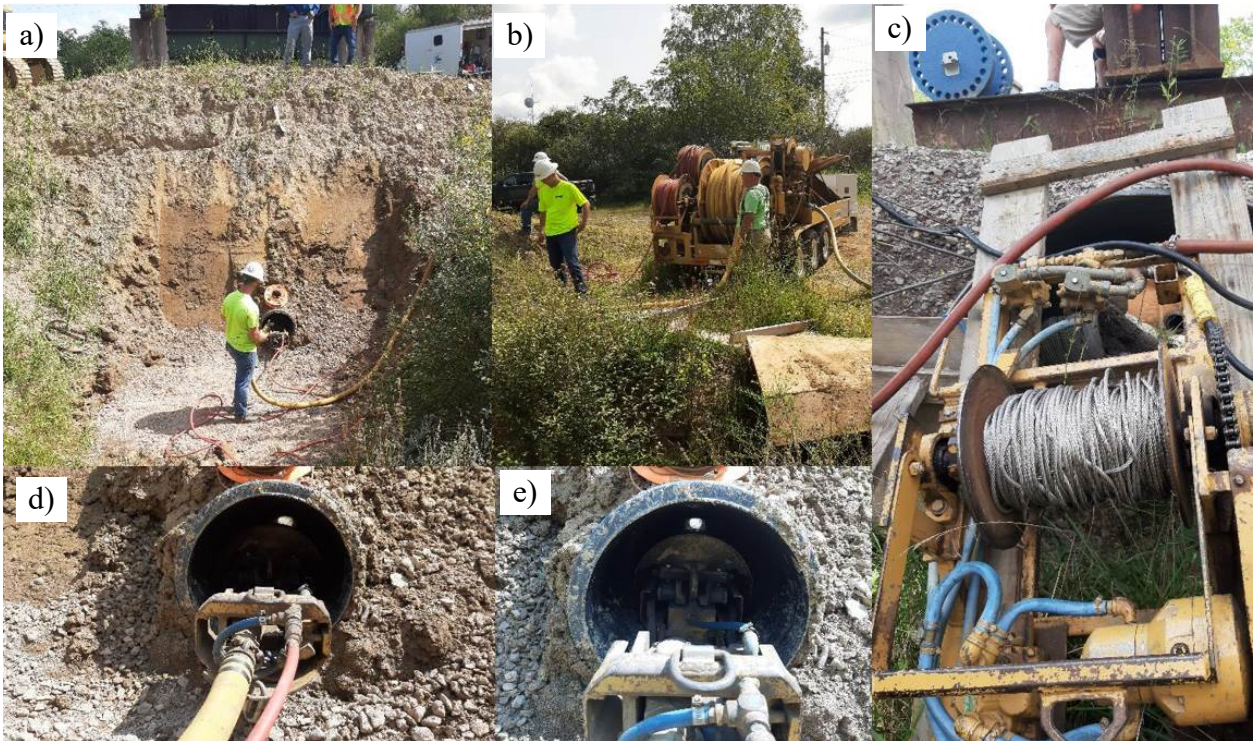
Figure 49. Views of re-rounding of Test Pipe 4: a) Re-rounder and operator at inlet of pipe; b) Reels with pneumatic and electrical cables connected to re-rounder; c) Winch at outlet to pull re-rounder through pipe; d) and e) Close-up views of re-rounder inside pipe.
