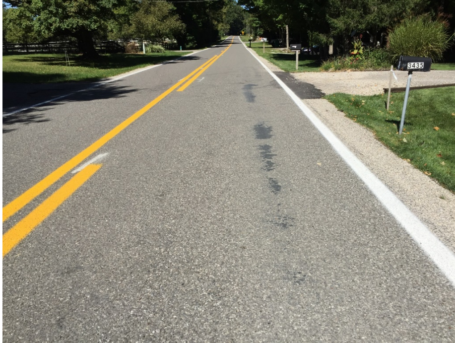
Figure D.2: Bleeding at the Transition between Pavement Sections 1 and 2 at the Franklin County Test Site.
