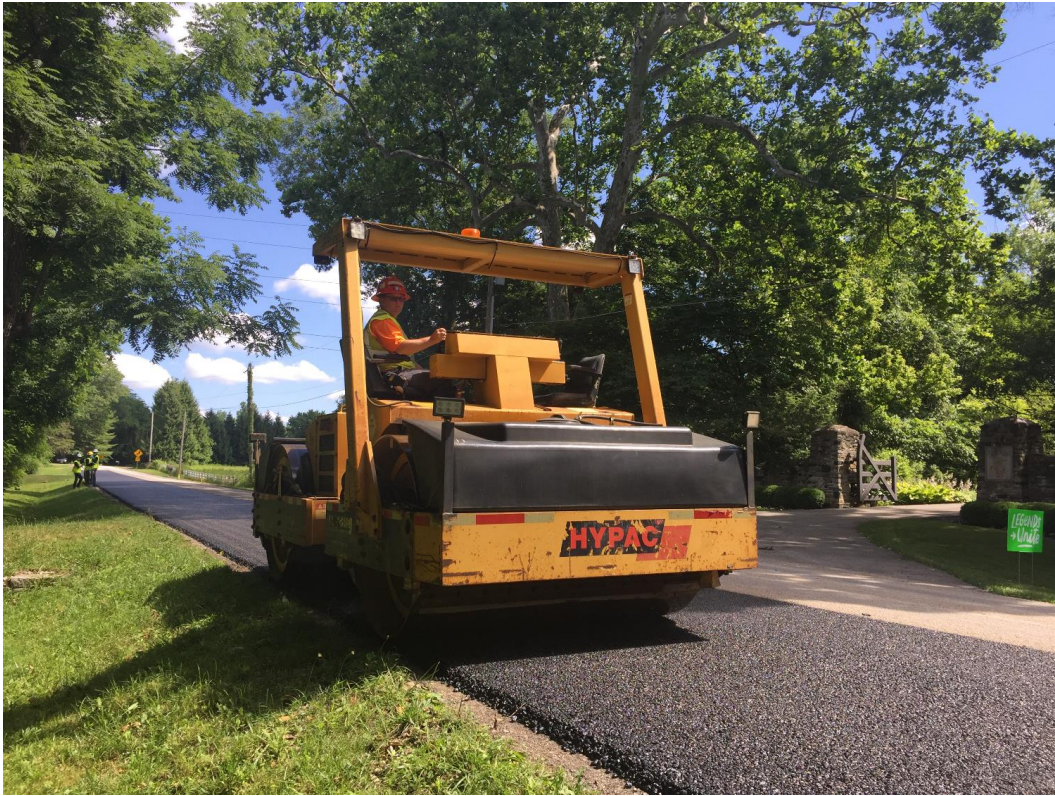
Figure A.5: Compaction of Asphalt Mixture at the Franklin County Test Site.
