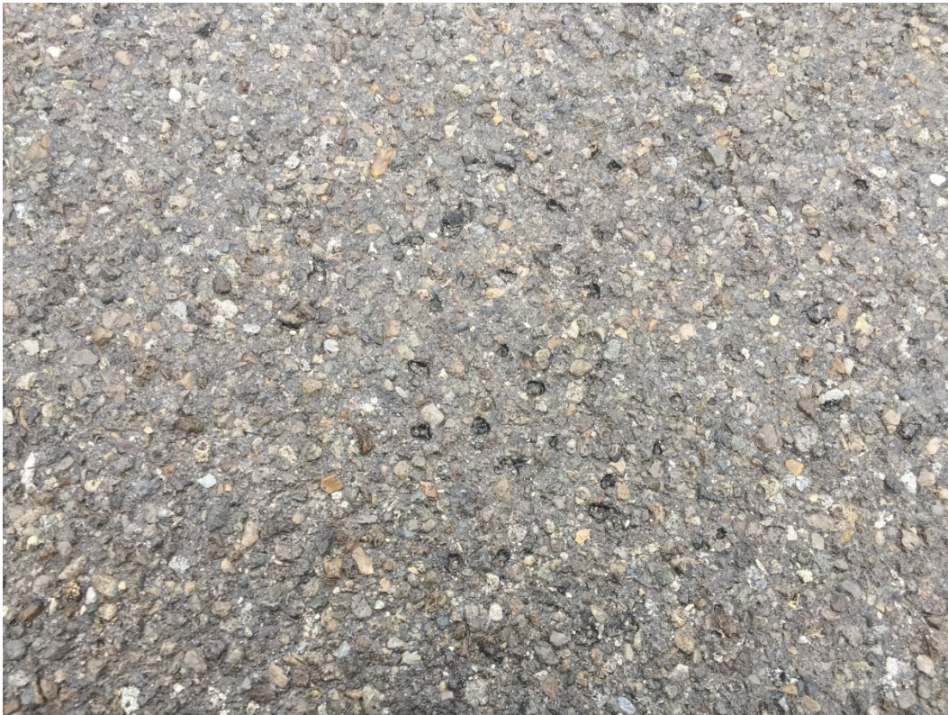
Figure D.4: Limited Aggregate Loss from the Chip Seal Layer at the Medina County Test Site.
