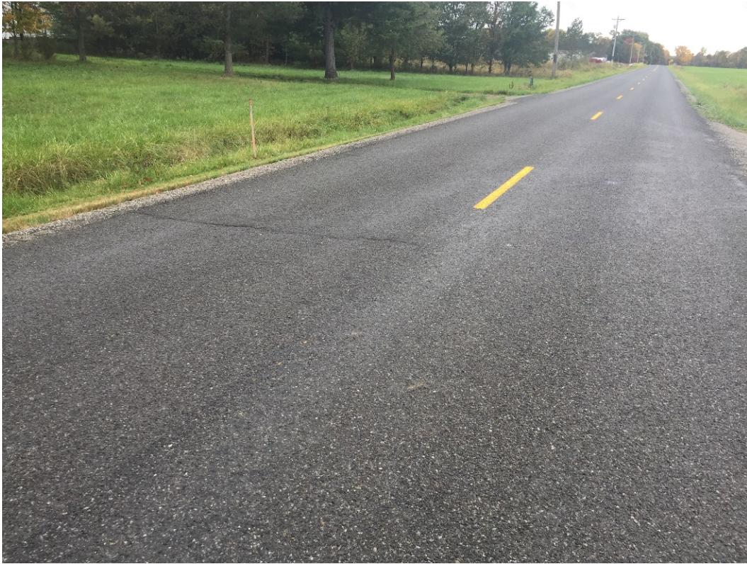
Figure D.5: Transverse Marks at the Medina County Test Site at the Transition between Pavement Sections or Interruption in Paving due to Rain.
