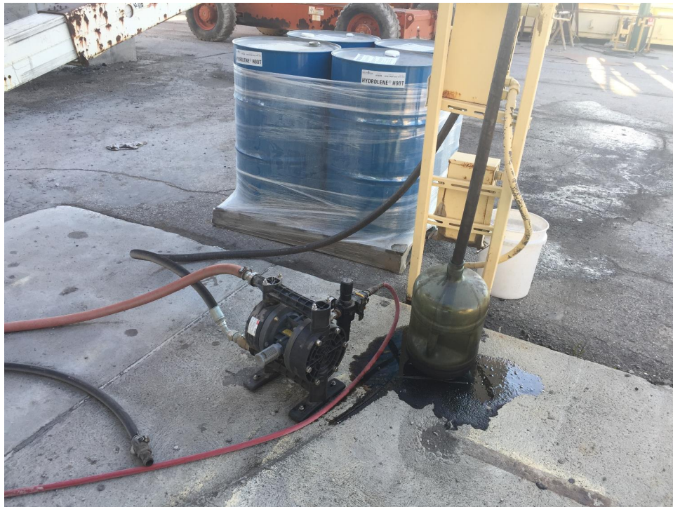
Figure A.3: Introduction of Aromatic Oil into the Asphalt Binder Line at the Asphalt Plant in Franklin County.
