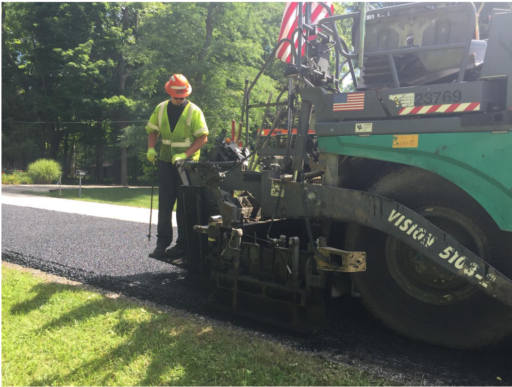
Figure A.4: Placement of Asphalt Mixture at the Franklin County Test Site.
