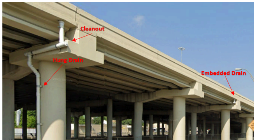
Figure 5.4 Hung and Embedded Systems Cleanout Plugs in Houston
