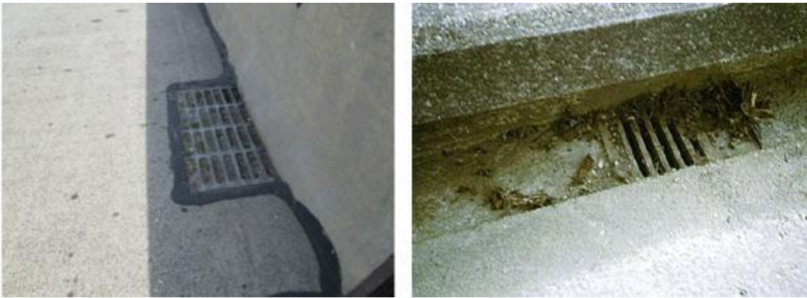
Figure 2.1 Clogging of bridge deck drain (FHWA, 2015; Zealand, 2011)
