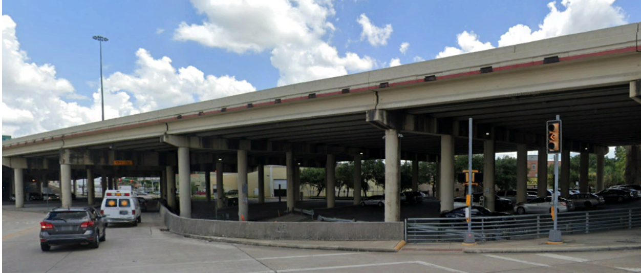
Figure 5.2 Free-fall Discontinues Over a Roadway in Houston
