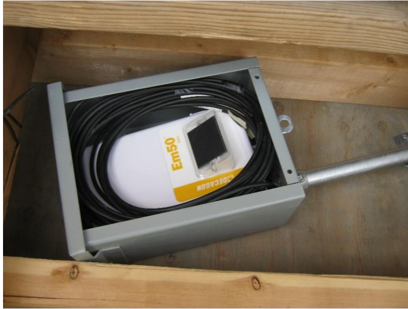
Figure 3-3 Data logger mounted inside a junction box.
