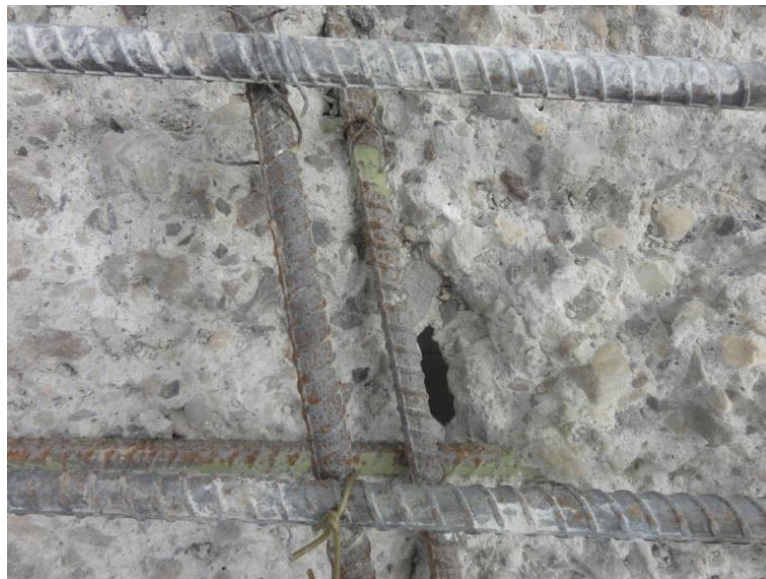
Figure 4-19: Insignificant blow-through of the deck in case study #2.
