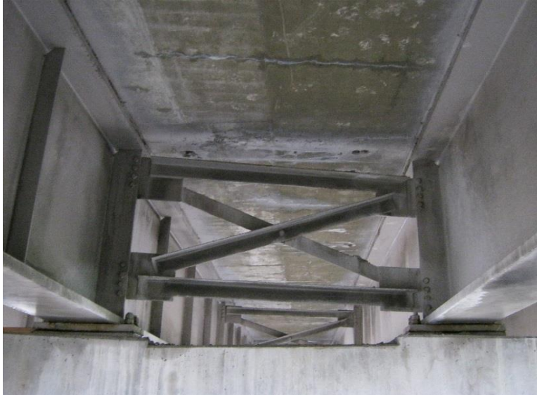
Figure 4-20: Insignificant efflorescence and cracking on the underside of the deck in case study #2.
