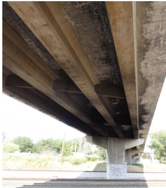
Figure 4-17: Significant efflorescence and cracking on the underside of the deck in case study #1.
