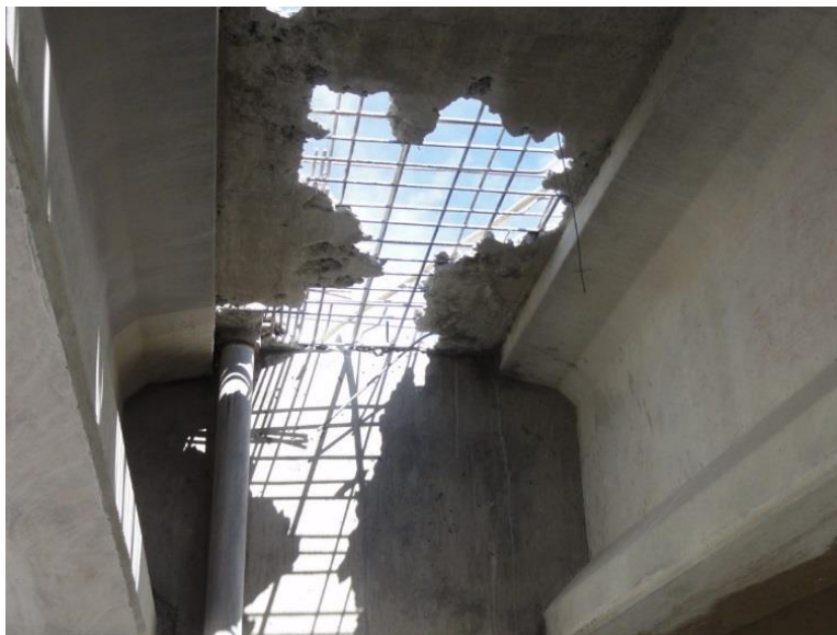
Figure 4-16: Significant blow-through of the deck in case study #1.
