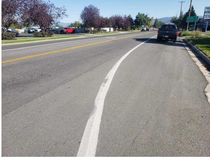
Figure 5-3 Section UT-04 Showing Some Joint Opening
