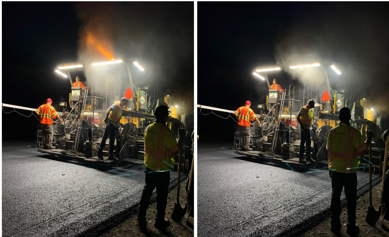
Figure 3.1: Paver with flashing amber lights on (left) and amber lights off (right) (case studies 1 and 3)
