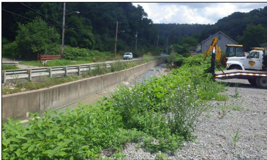
Figure B-2: Looking downstream along Streets Run with SR 2046 beyond the left banks. PennDOT photo
