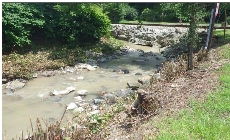
Figure B-3: Looking downstream along Streets Run from Corley Street Bridge. PennDOT photo
