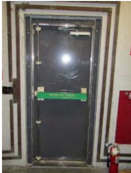
Figure 15 - Example of Permanent Flood Door (Credit: MassDOT)
