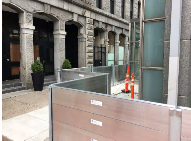
Figure 22 – Southwest Headhouse Flood Barriers (Credit: MassDOT)
