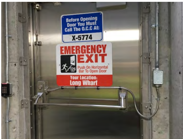
Figure 19 – Long Wharf Flood Door - Interior (Credit: MassDOT)
