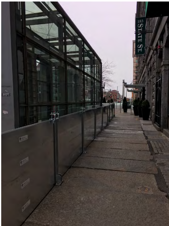
Figure 23 – Southwest Headhouse Flood Barriers (Credit: MassDOT)
