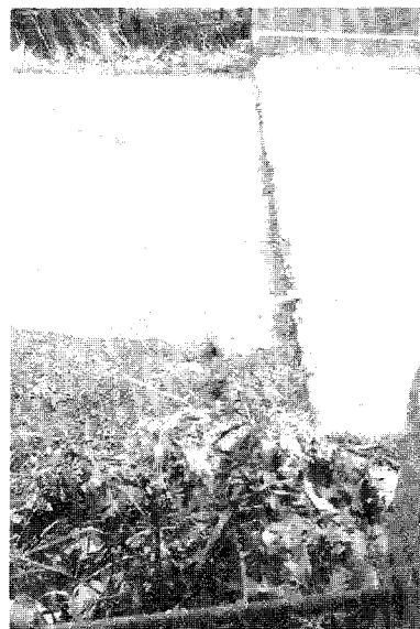
Slide No. 6-3-8 Example Slide Heaving of the approach pavement
