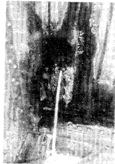
Slide No. 6-1-49 Example Slide Deteriorated stay-in-place form
