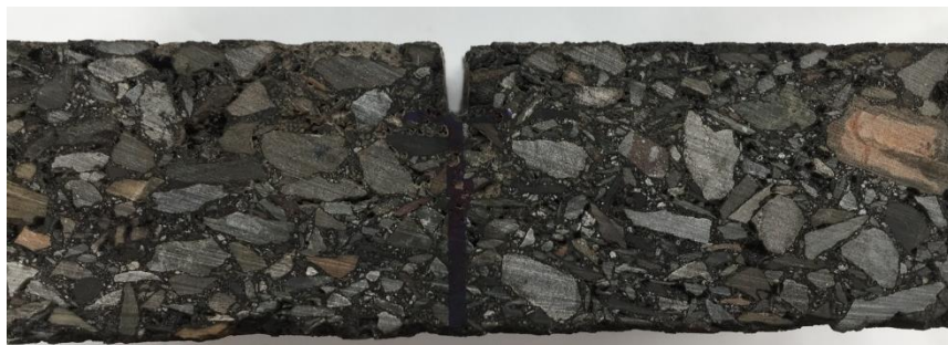
Figure 11. Distressed HMA Sample.
