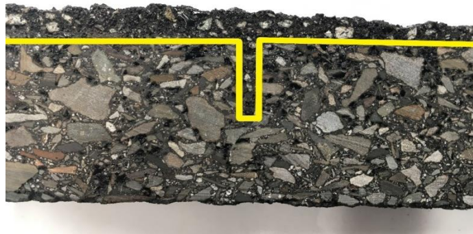
Figure 16. Microsurface Presence in 3mm Crack.
