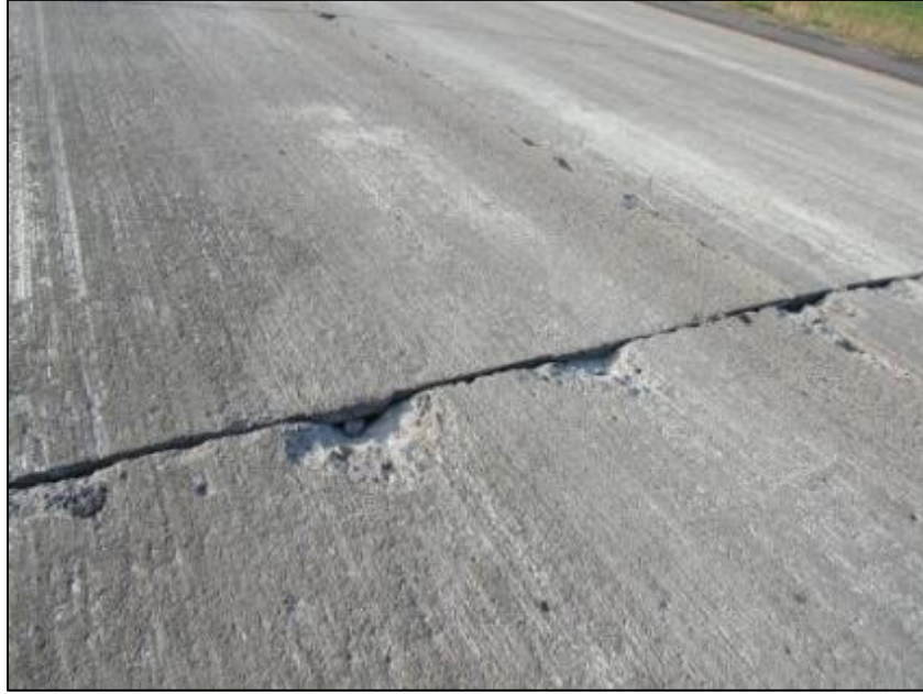
Figure 3-9. Spalling in Cell 506 (control, non-FRC) observed in the year 2018.
