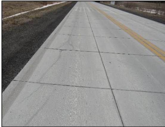
Figure 3-6. Longitudinal cracks in Cell 239 (April 2019).
