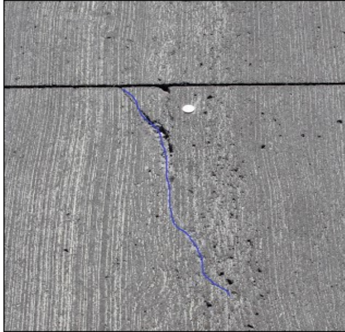
Figure 3-22. Longitudinal crack in Cell 805 (2018)
