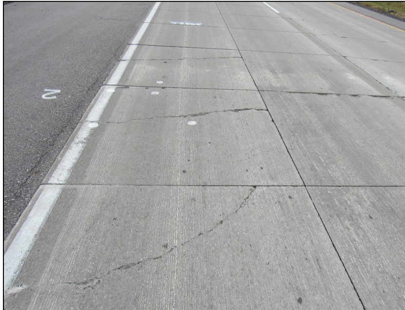
Figure 3-10. Photographs of transverse and diagonal cracks in Cell 506 (October 2019).
