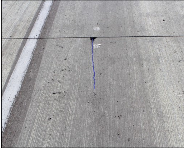
Figure 3-17. Longitudinal crack in Cell 705 (2018).
