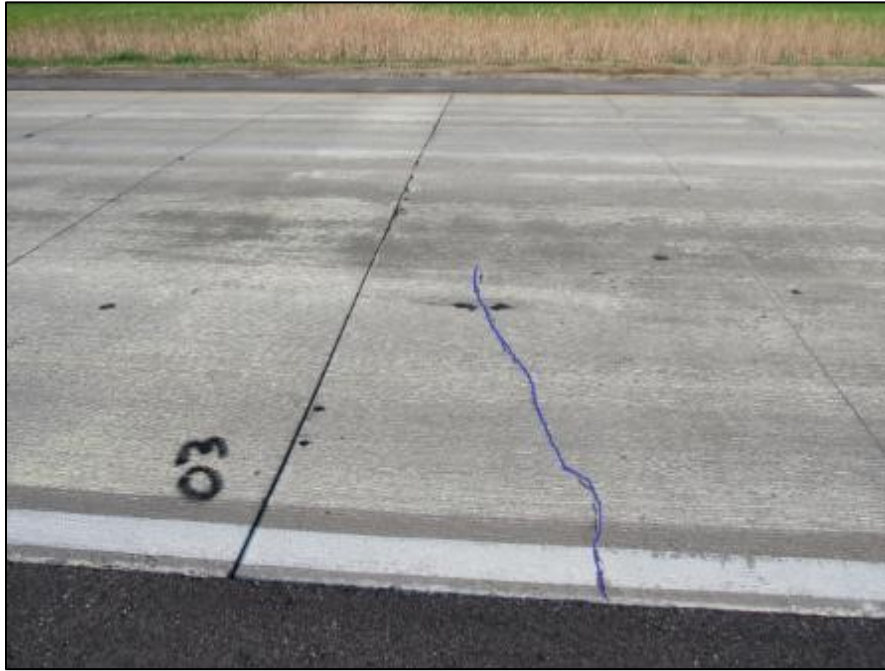
Figure 3-8. Transverse crack in Cell 506 (control, non-FRC) observed in the year 2018.
