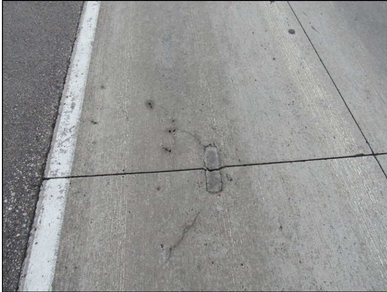
Figure 3-15. Narrow cracks in Cell 806, originated at the location of the joint opening sensor.
