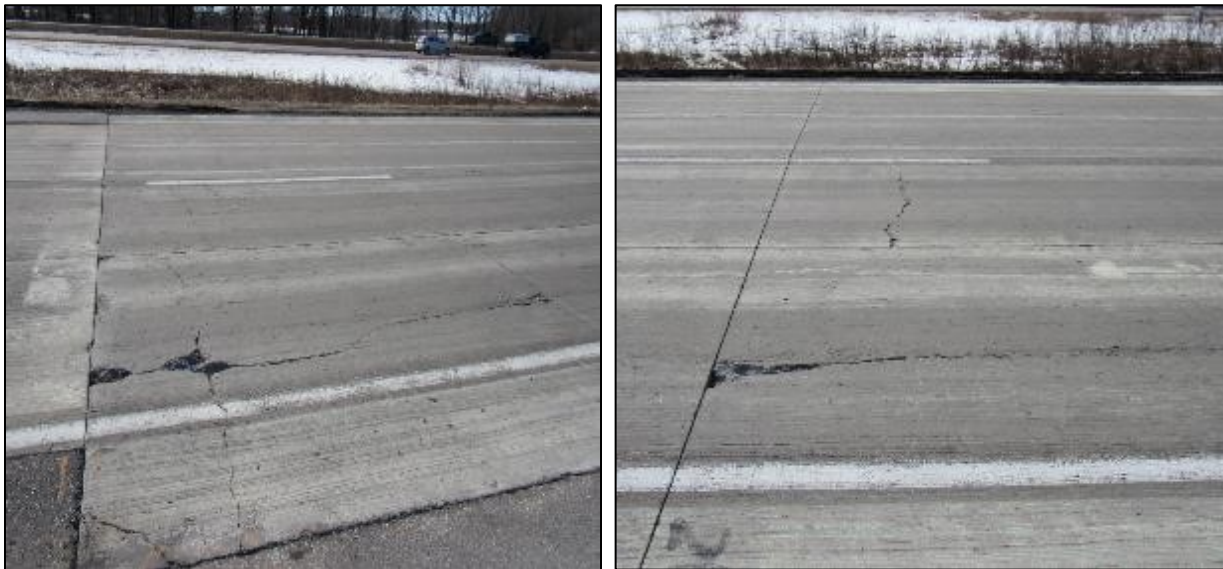
Figure 3-25. Photographs of observed cracks in Cell 805 during April 2019.
