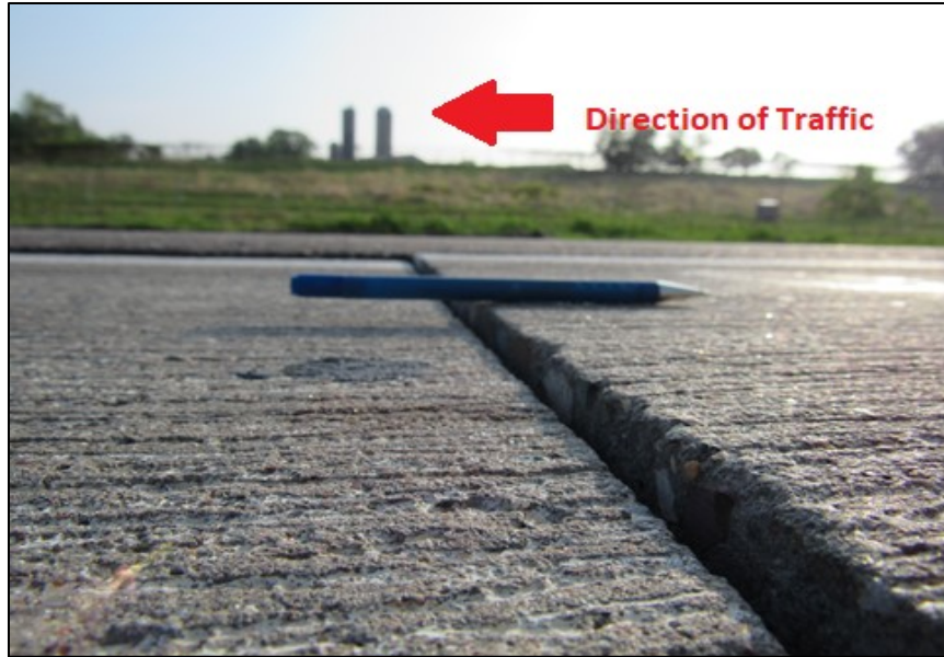
Figure 4-3. Photograph of faulting of Cell 506 (non-FRC). Note that the faulting shown in this photograph is exaggerated due to the broken corner in the slab on the leave slab.
