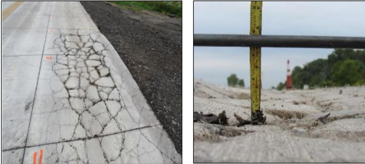
Figure 3-2: Shattered slabs and depression along the wheel path in Cell 139 after MnROAD truck loadings.
