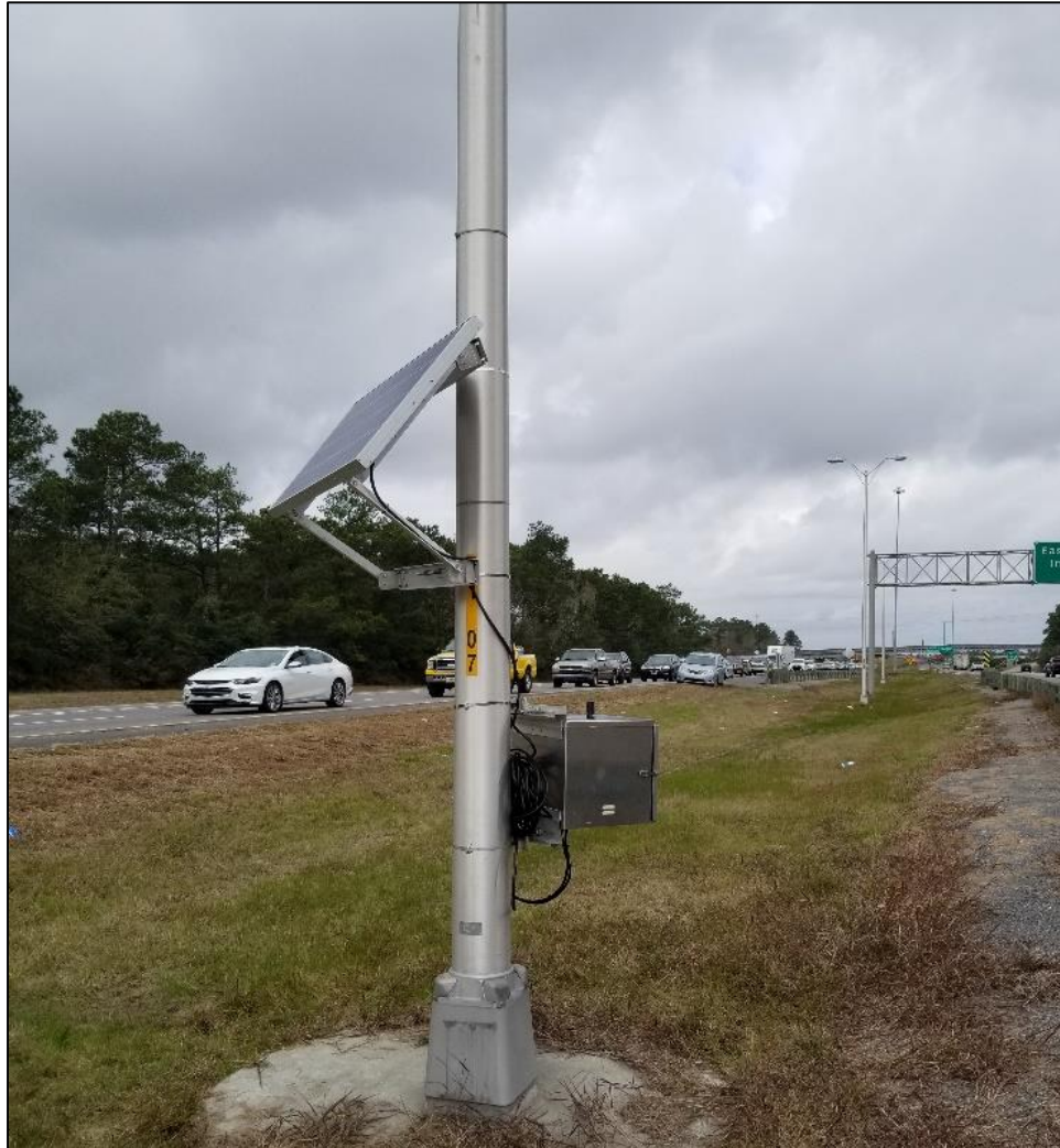
Figure 30. Solar panel serves as source of power for RTMS device
