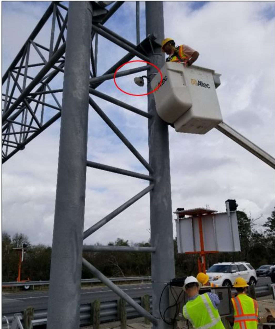
Figure 29. Installation of RTMS device (circled)
