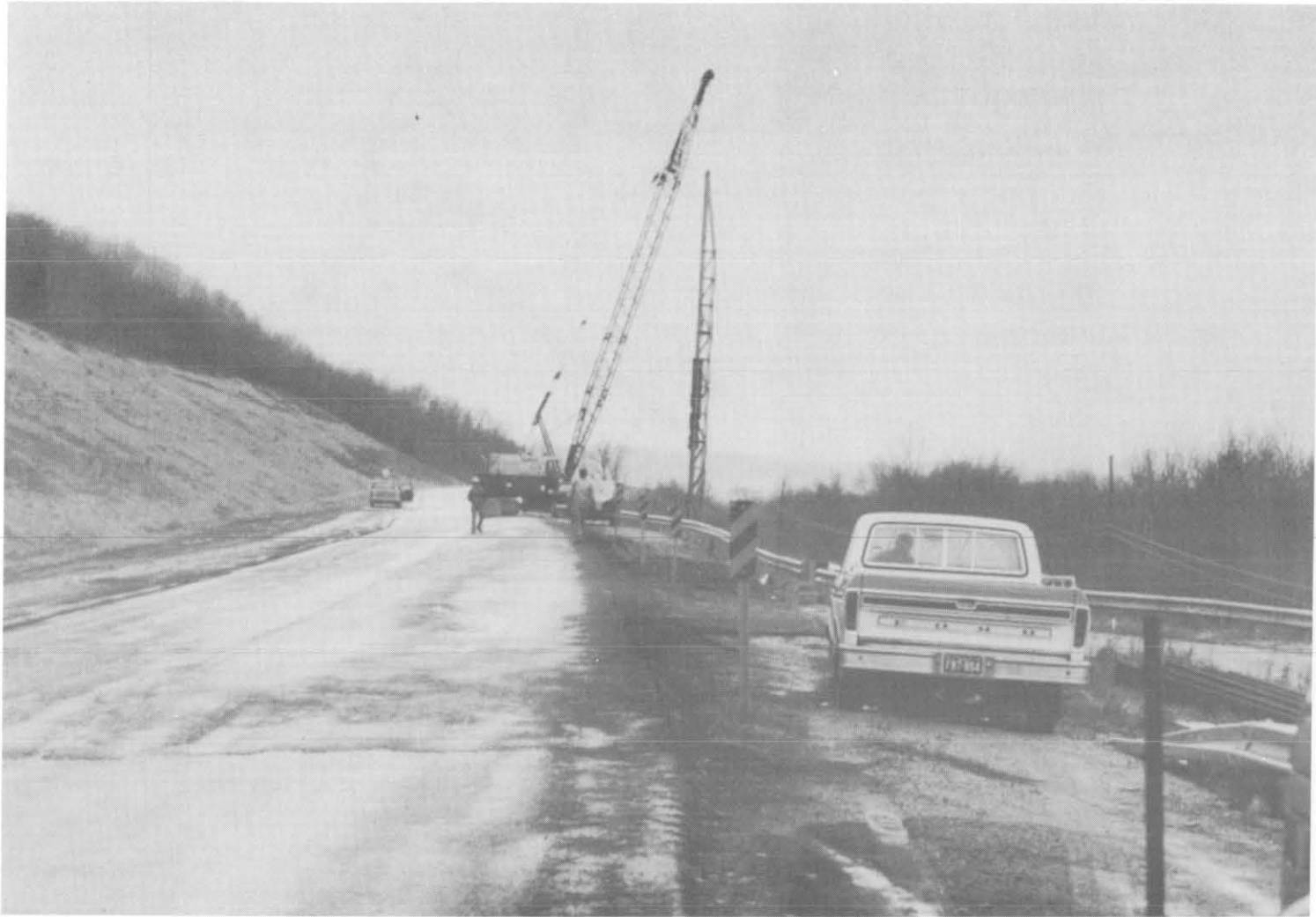
Figure 1. Ky. 227 Slide Site Prior to Remedial Action.
