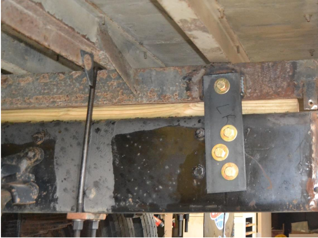
Left-Rear Shear Plate and U-Bolt
