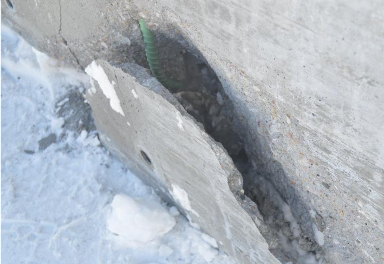
Figure 225. System Damage, Concrete Damage at Post No. 9, Test No. STBR-2
