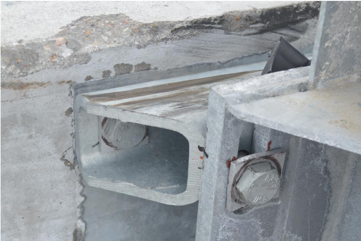
Figure 271. System Damage, Concrete Damage at Post No. 7 Location, Test No. STBR-3
