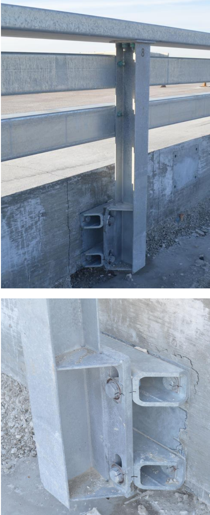
Figure 170. Post No. 8 Damage, Test No. STBR-1
