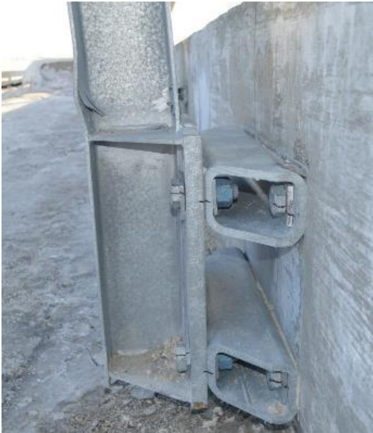
Figure 169. Post No. 7 Damage, Test No. STBR-1 233
