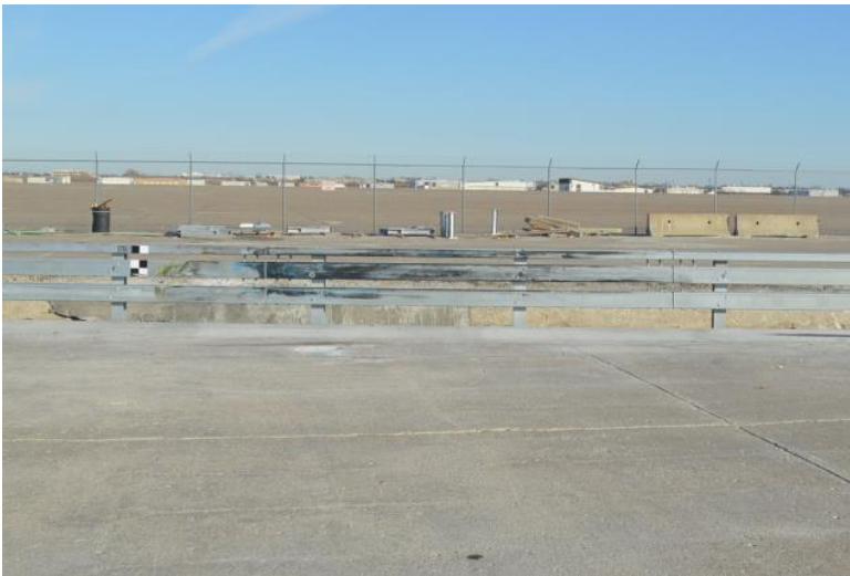
Figure 165. System Damage, Test No. STBR-1
