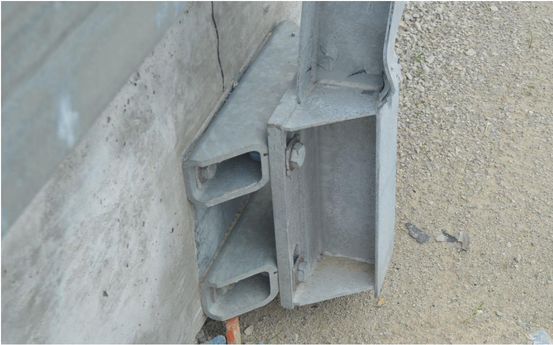
Figure 324. System Damage, Post No. 6, Test No. STBR-4
