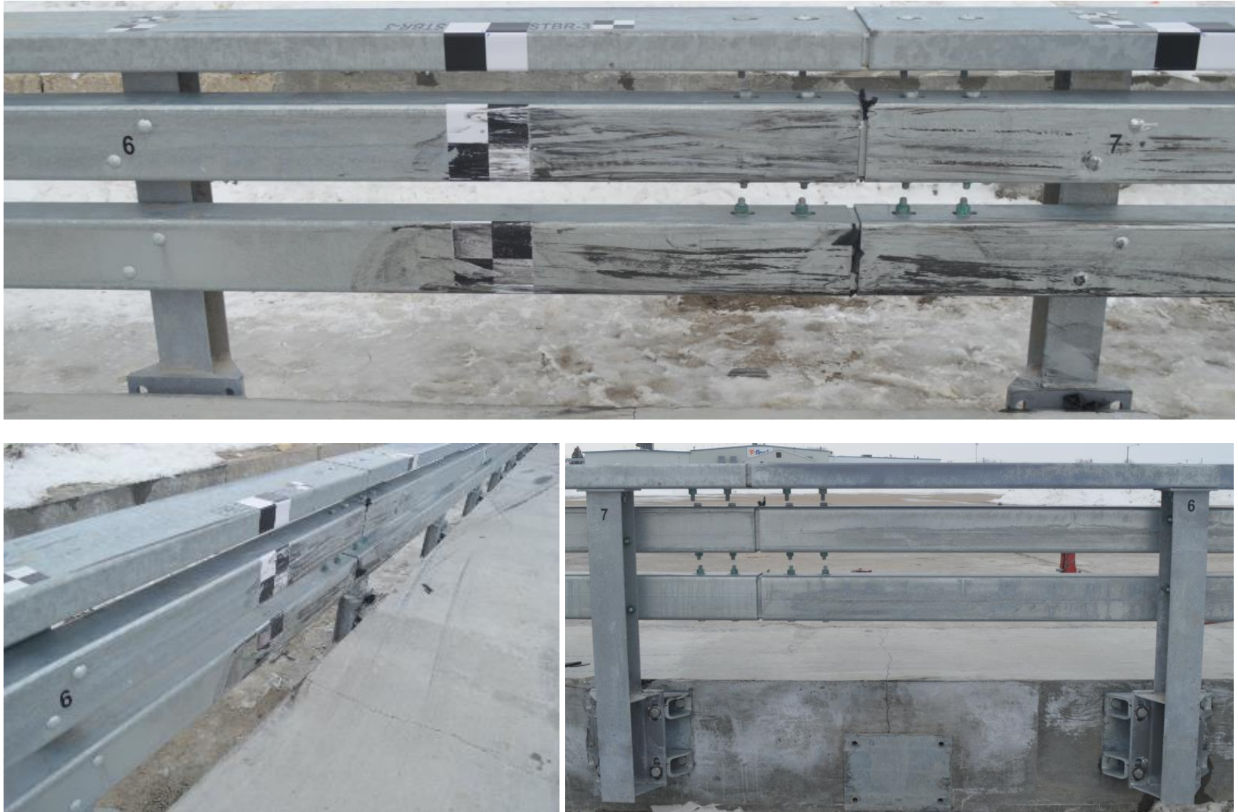
Figure 269. System Damage, Rail Span Between Posts Nos. 6 and 7, Test No. STBR-3
