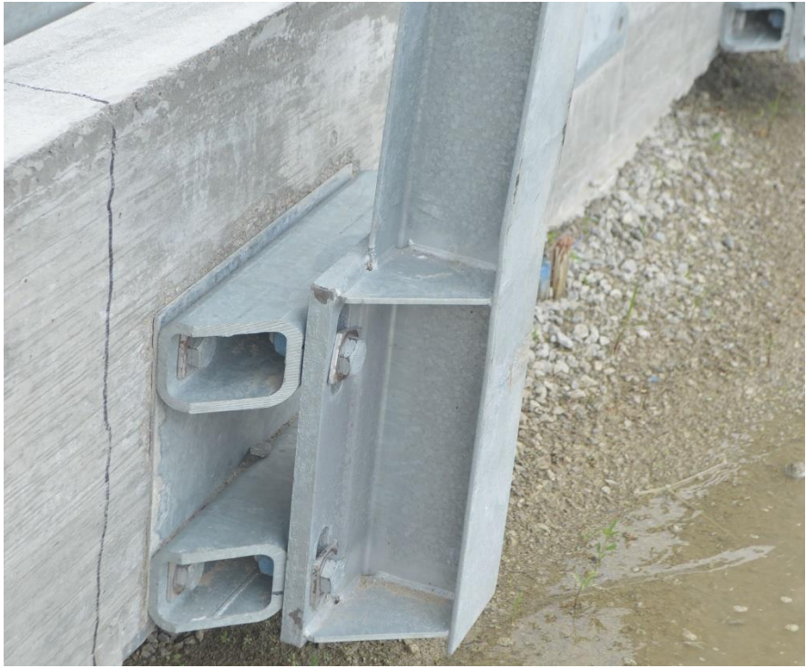
Figure 326. System Damage, Post No. 8, Test No. STBR-4
