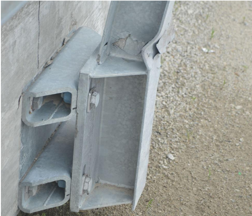
Figure 325. System Damage, Post No. 7, Test No. STBR-4
