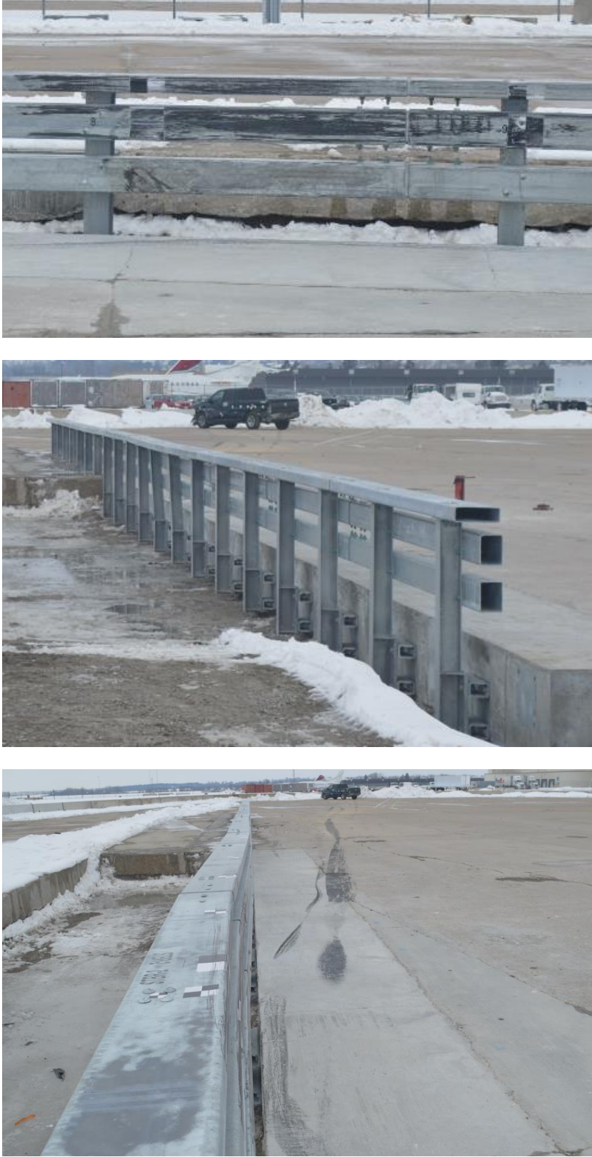
Figure 218. System Damage, Test No. STBR-2
