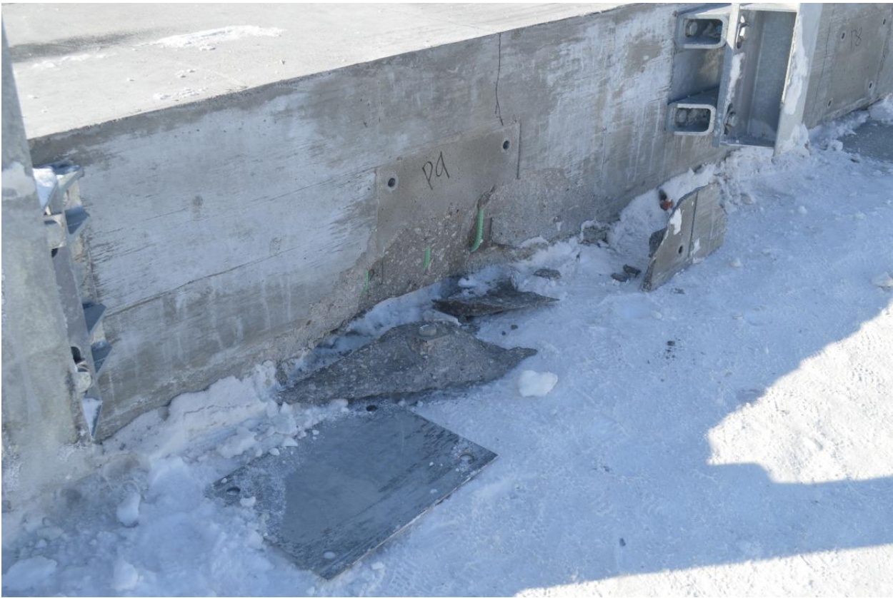
Figure 226. System Damage, Concrete Damage at Post No. 9, Test No. STBR-2
