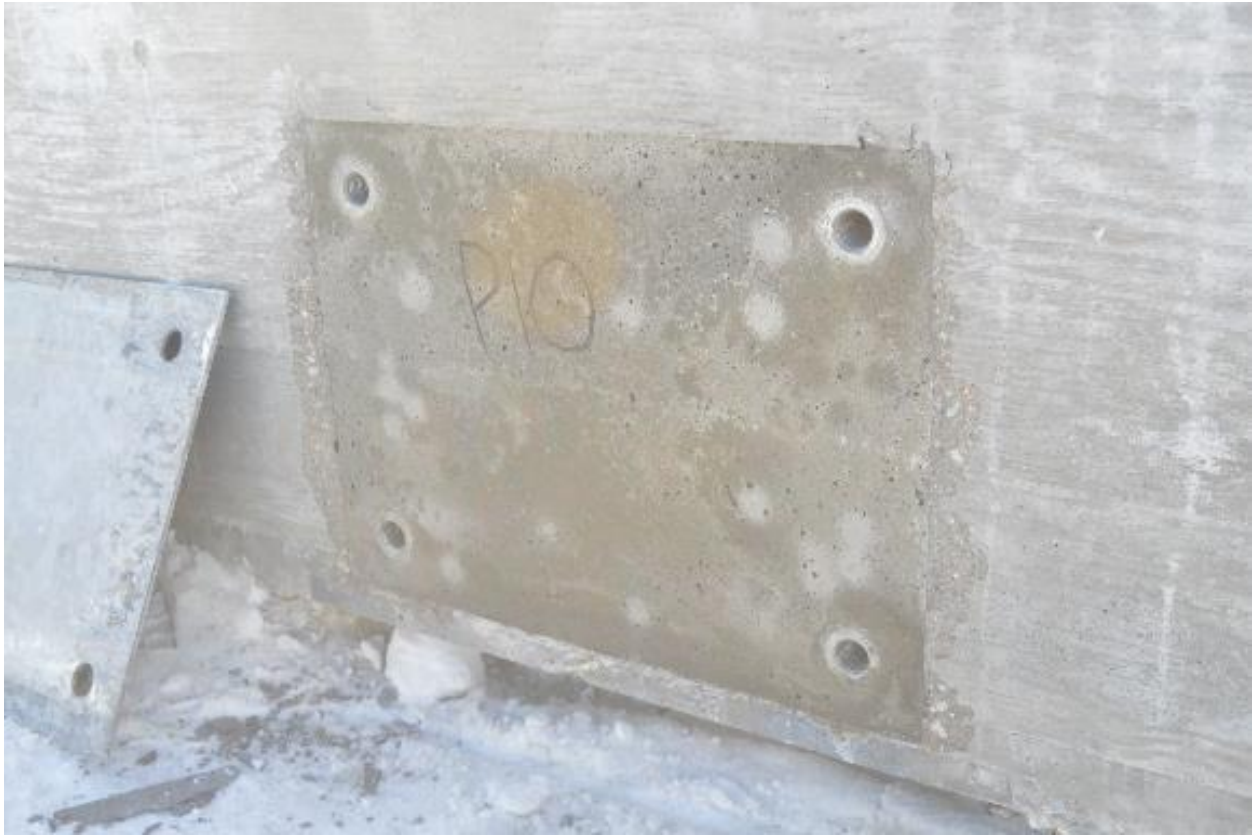
Figure 227. System Damage, Concrete Damage at Post No. 10, Test No. STBR-2
