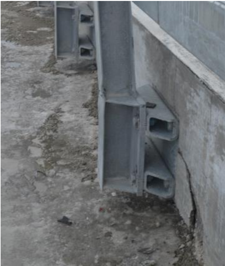
Figure 223. System Damage, Post No. 9, Test STBR-2
