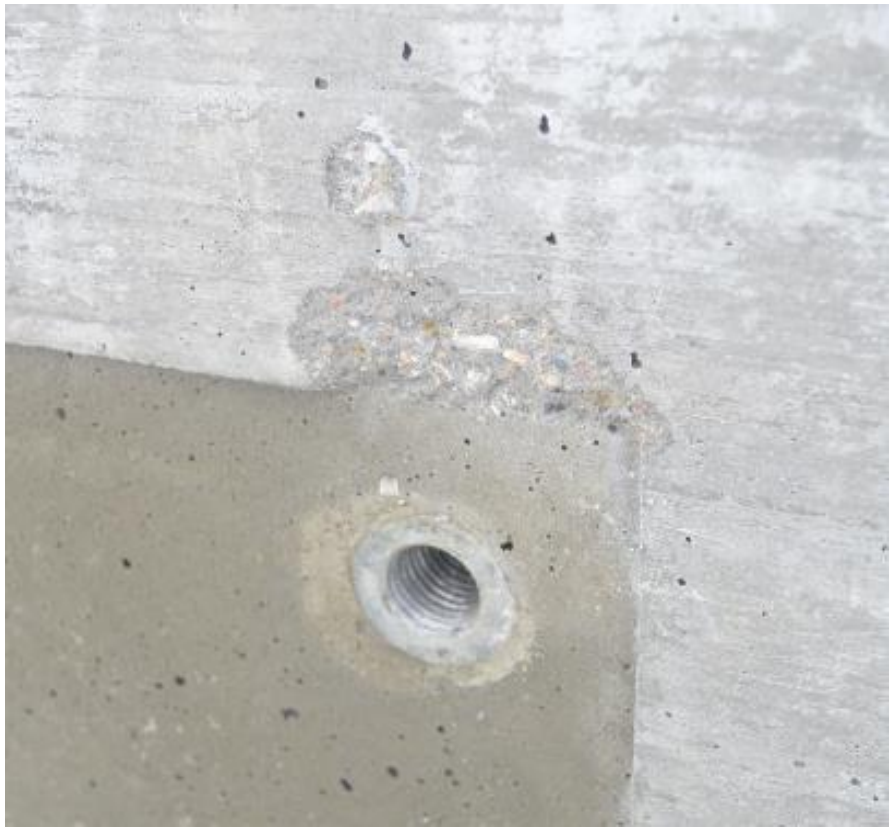
Figure 171. Concrete Damage at Post No. 7, Test No. STBR-1
