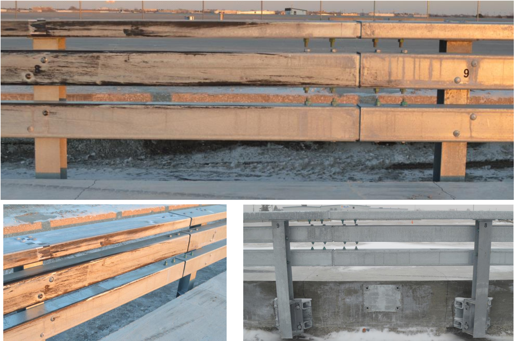
Figure 168. Damage to Rail Span Between Posts Nos. 8 and 9, Test No. STBR-1
