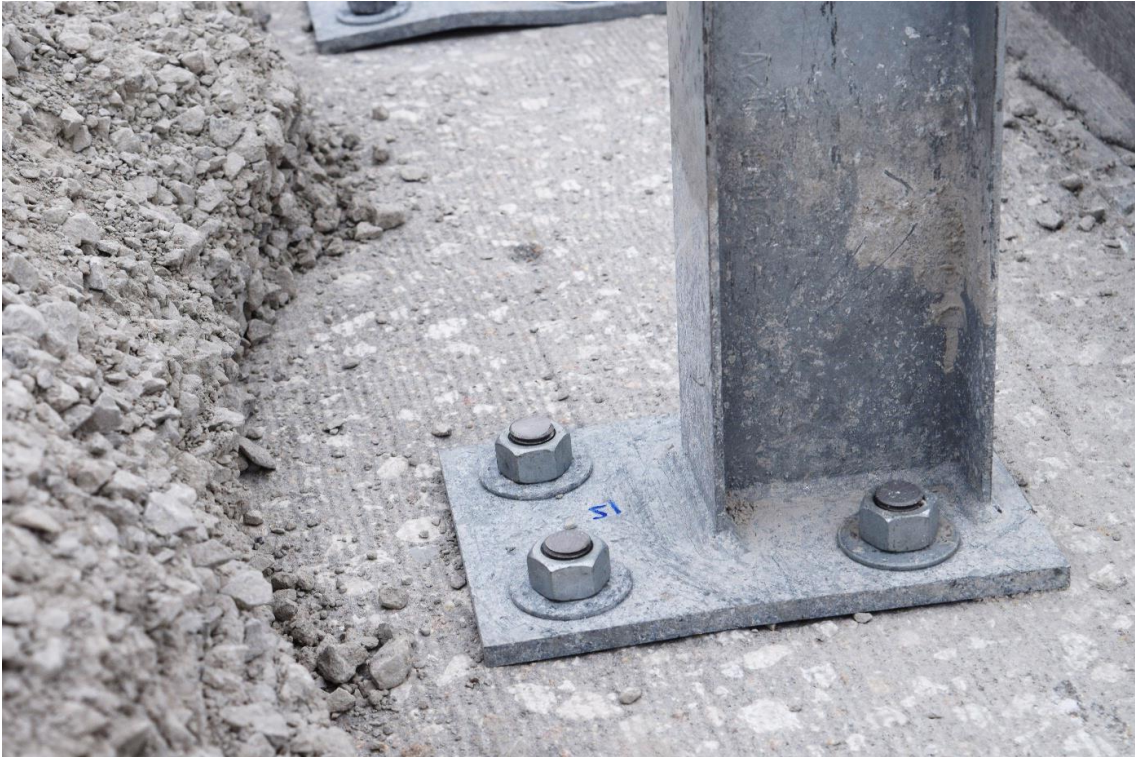
Figure 64. Damage to Post and Base Plate No. 21, Test No. CMGS-1
