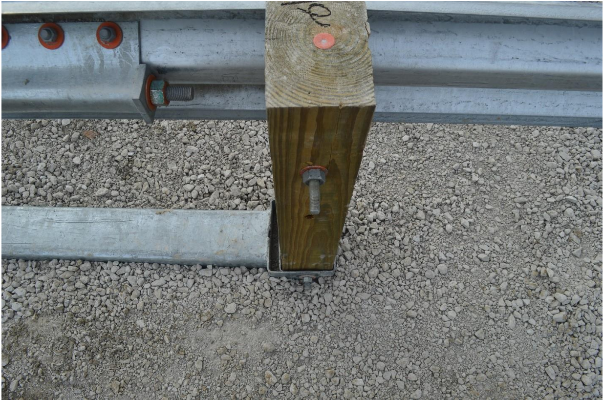
Figure 89. Damage to Upstream Anchorage System, Test No. CMGS-2
