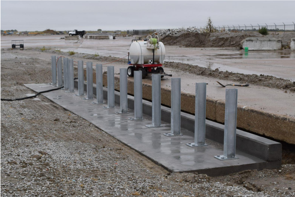
Figure 21. Concrete Culvert Superstructure, Top Slab, Headwall, and Vertical Supports, Test Nos. CMGS-1 and CMGS-2
