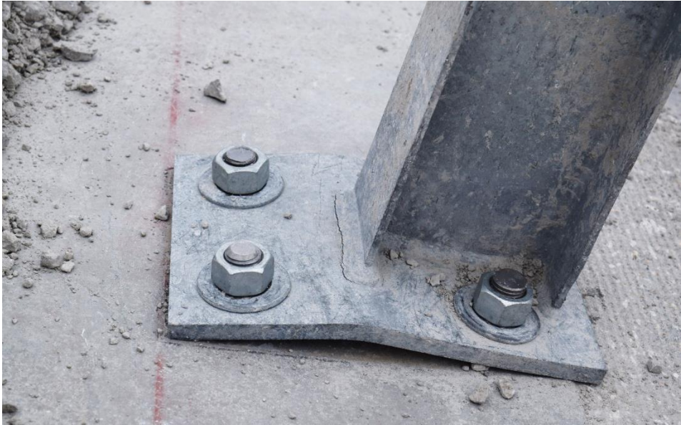
Figure 62. Damage to Post and Base Plate Nos. 17 through 21 (After Removal of Soil Fill Post and Base), Test No. CMGS-1
