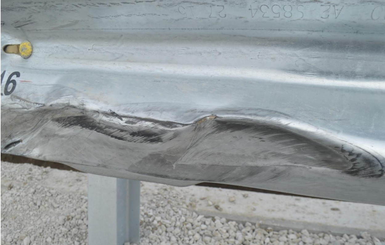
Figure 84. Rail Tears at Post No. 16, Test No. CMGS-2
