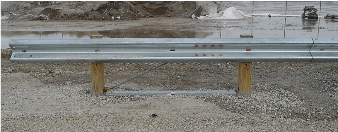
Figure 88. Culvert Deck after Removal of Soil Fill and Posts and Downstream Anchorage System Deformation, Test No. CMGS-2
