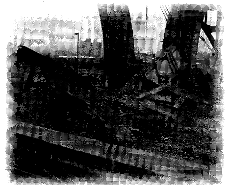
After demolition, the steel girders were extracted from the wreckage and sent to TFHRC for evaluation.
