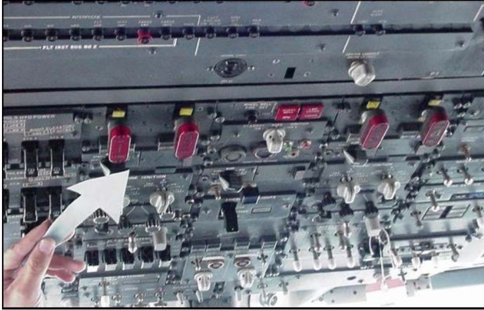
Figure 51. The B-747 Fire Handles (Photograph courtesy of IPA)
