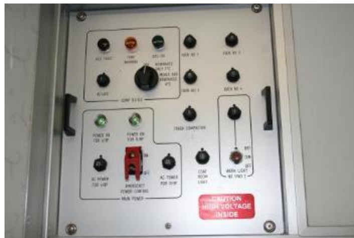
Figure 103. Galley Electrical Panel, Including Emergency Power Shutoff (Photograph courtesy of FAA)
