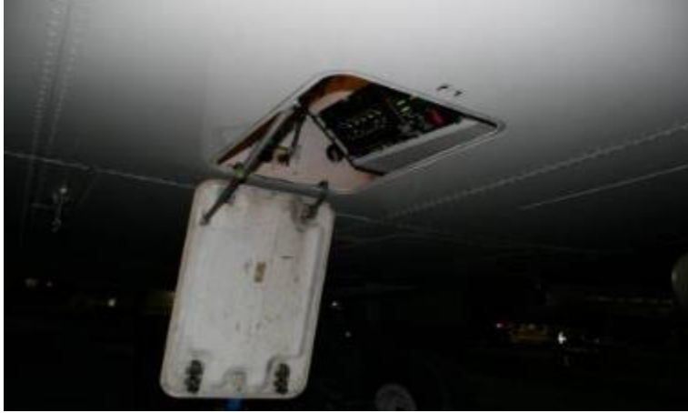
Figure 168. Refuel/Defuel Panel (Photograph courtesy of FAA)
