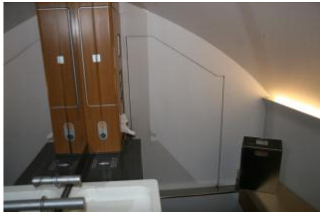
Figure 75. Access Point to A380 Upper-Deck Avionics Through the Lavatory (Photograph courtesy of FAA)
