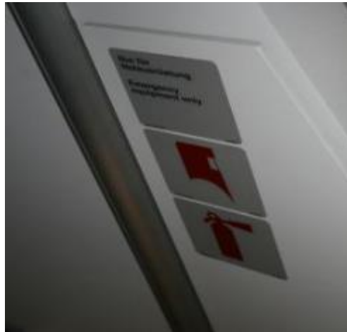
Figure 76. Typical Labels on Compartments Used to Store Fire Extinguishers and Hoods (Photograph courtesy of FAA)
