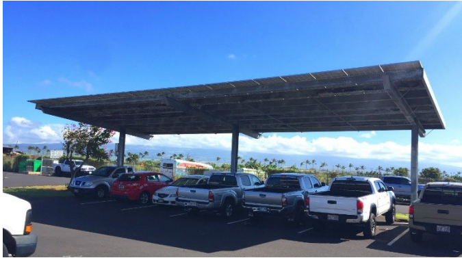
Solar canopy at a maintenance baseyard on Maui. (Image source: Hawaii DOT).
