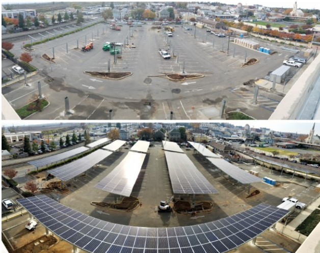
Installation of a solar canopy at a Caltrans parking lot (Image source: Caltrans).
