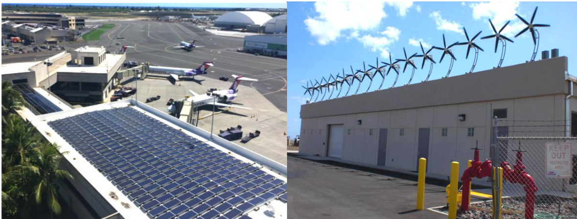
Figure 1: Solar panels and wind turbines at Honolulu International Airport (Image source: Hawaii DOT).
