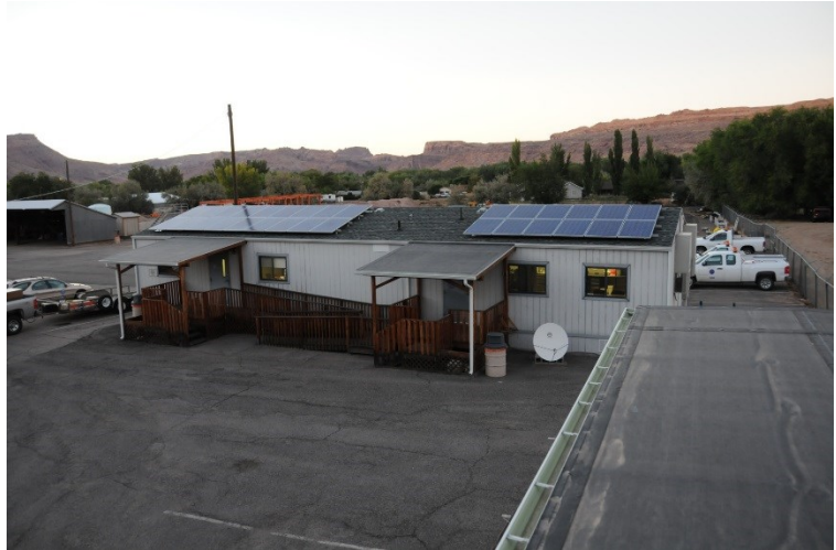
Solar panels on a UDOT construction office (Image source: UDOT).
