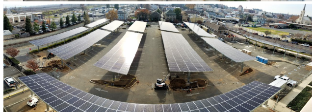
Figure 3: Installation of a solar canopy at a Caltrans parking lot (Image source: Caltrans).
