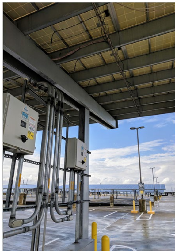
Figure 5: Solar canopies at BWI Airport in Baltimore, MD (Source: Volpe Center).
