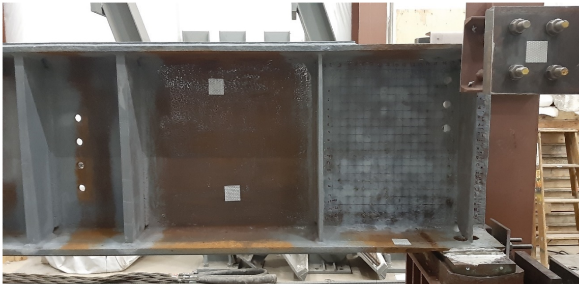
Figure 3.7: Corroded end of Specimen A
