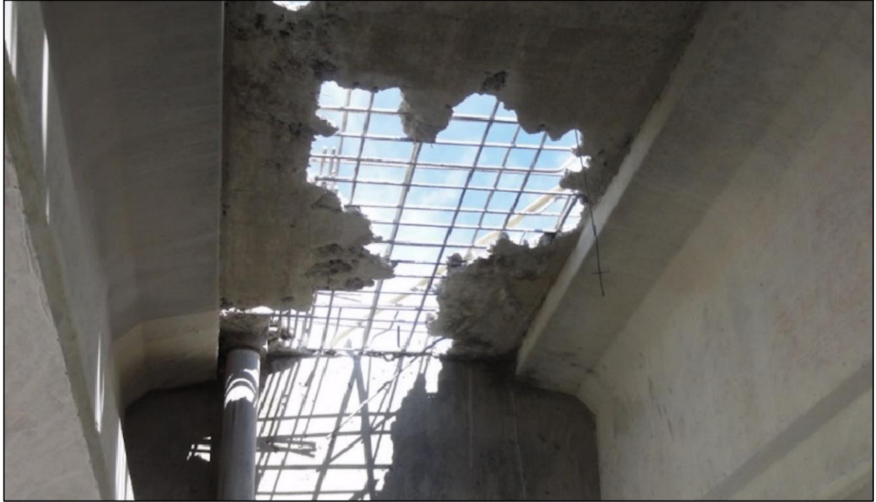
Figure 2.4.4.2 Severe Hydrodemolition Blow-Through (Roper 2018)
