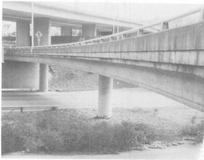
Figure 13. View of side of curved concrete box girder bridge shown in figure 12 showing no signs of distress in spite of the settlements that took place.
