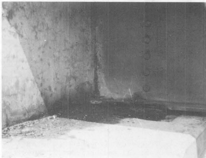
Figure 3. Backwall of abutment jammed against beam as result of inward horizontal movement of abutment.
