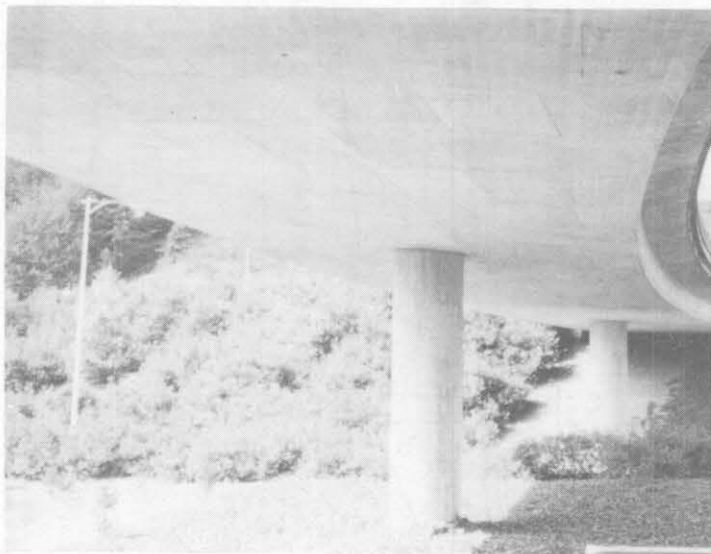
Figure 14. View of bottom of curved concrete box girder bridge shown in figures 12 and 13 showing no signs of distress in spite of the settlements that took place.
