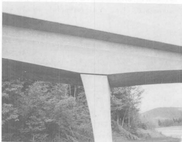
Figure 11. Closeup of bridge shown in figure 10 showing no signs of distress in spite of differential settlement of abutment.
