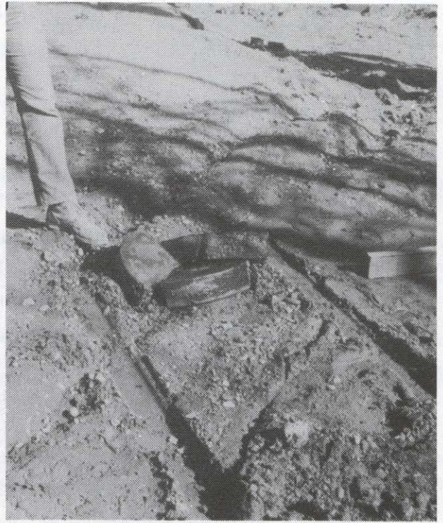
Figure 24.3 Damaged Hammer Cushion
