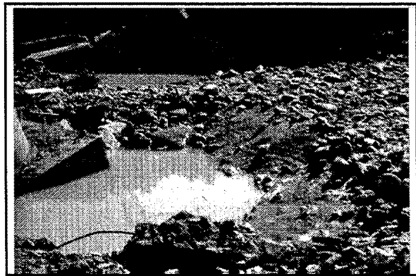
1.3 Schoharie Creek scour hole at pier 2
