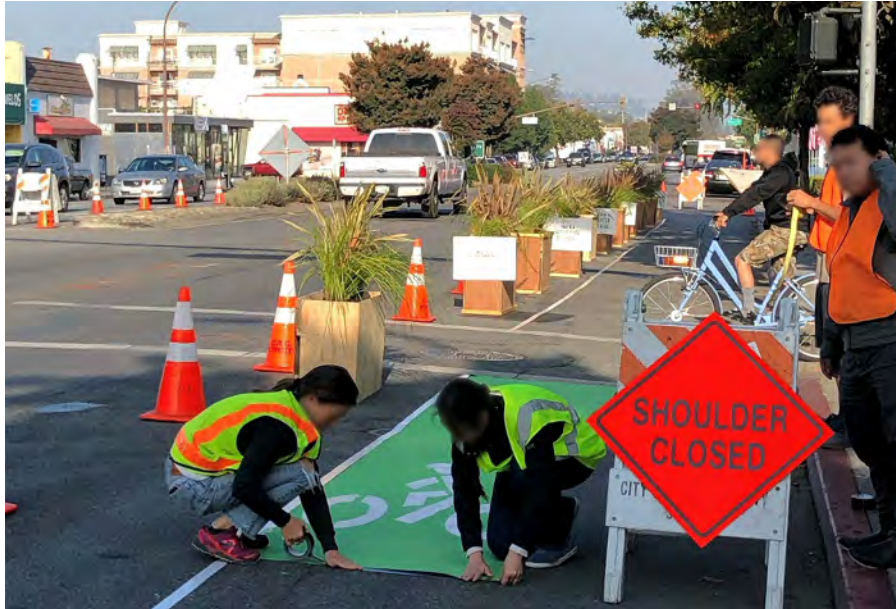
Figure 5. Photo. Living previews allow the short-term demonstration of new projects or concepts with temporary materials, such as this pop-up protected bike lane in Redwood City, CA, USA. Source: Fehr & Peers.
