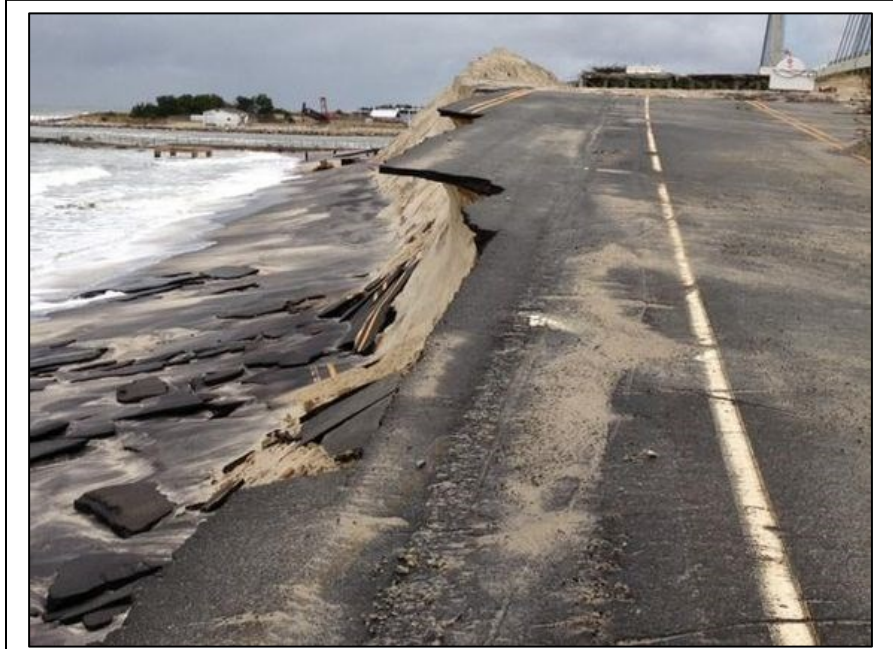
Figure 5 - Erosion from Hurricane Sandy that Affected SR 1 Near the Indian River Inlet Bridge. Source: DNREC, 2012.
