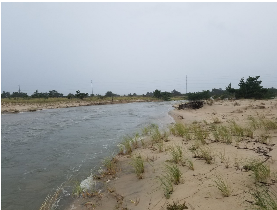
Figure 13 – Breach of Eastern Dune System at Conquest Road on September 19, 2017. Source: DelDOT
