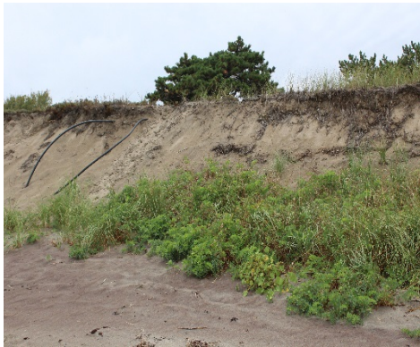
Erosional scarp at Route 209 shoulder Phippsburg, ME; September 19, 2016 Credit: Maine DOT
