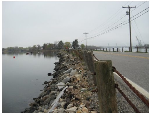
US Route 1B Causeway New Castle, NH; May 4, 2011 Credit: New Hampshire DOT
