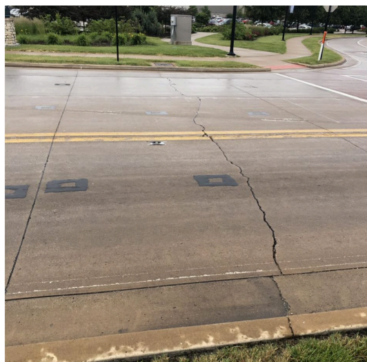
Figure 18. Photo. MacArthur Highway transverse distress near utility duct.
