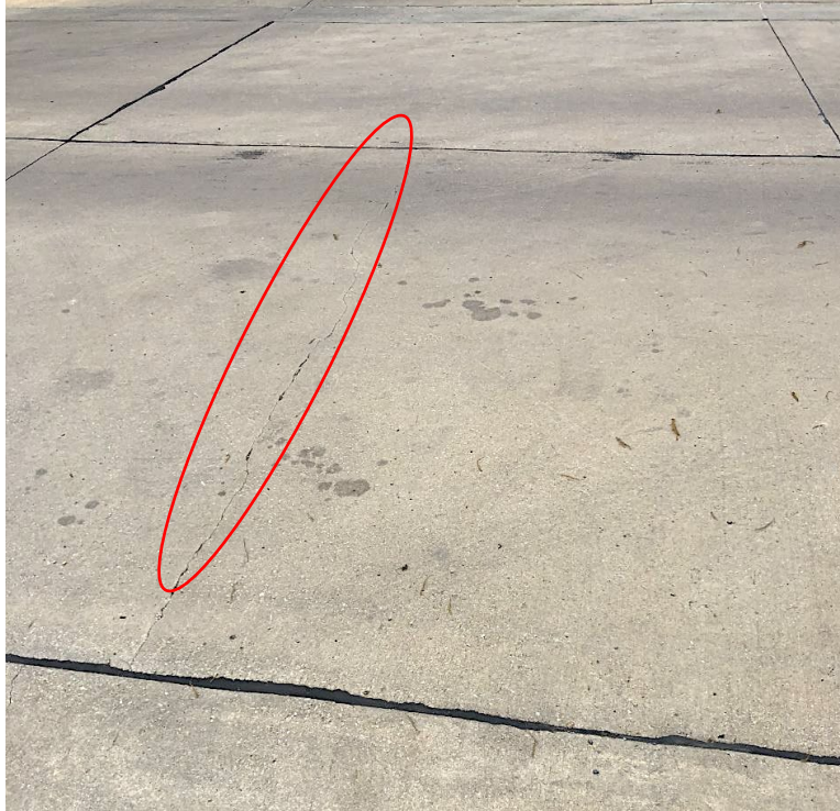
Figure 21. Photo. Healey Street premature mid-panel crack.
