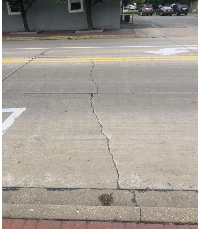
Figure 19. Photo. Transverse crack on Jefferson Avenue near Jackson Street.
