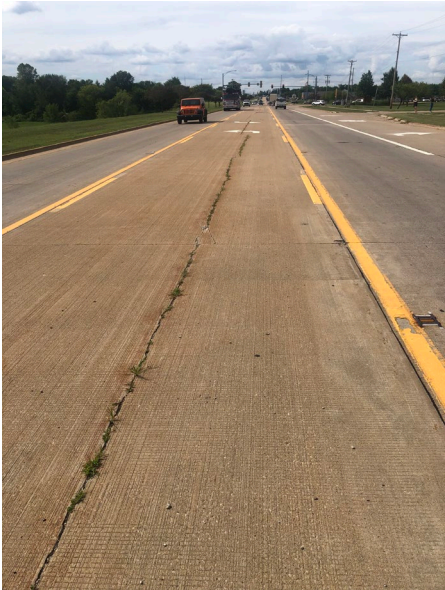
Figure 13. Photo. US 20 longitudinal cracking in a two-way left turn lane.
