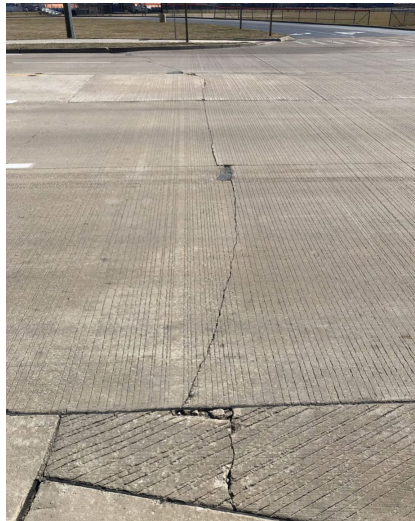
Figure 16. Photo. IL 71 transverse cracking distress.
