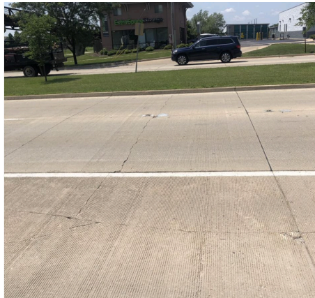
(B) IL 59 section constructed in 1998 (significant cracking).
