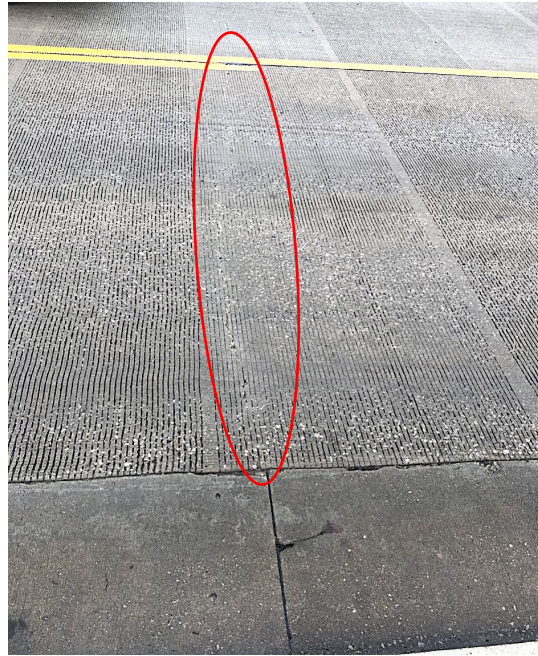
Figure 23. Photo. Harrison Street transverse crack.
