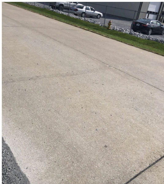
Figure 25. Photo. Mid-panel transverse crack on Central Street (East St. Louis, IL).
