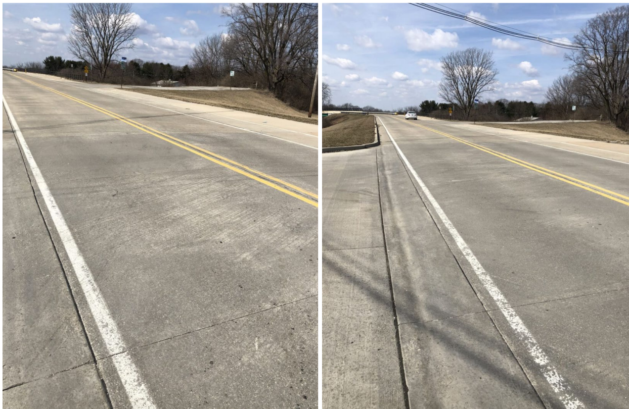
Figure 94. Photos. Lake of the Woods Road.
