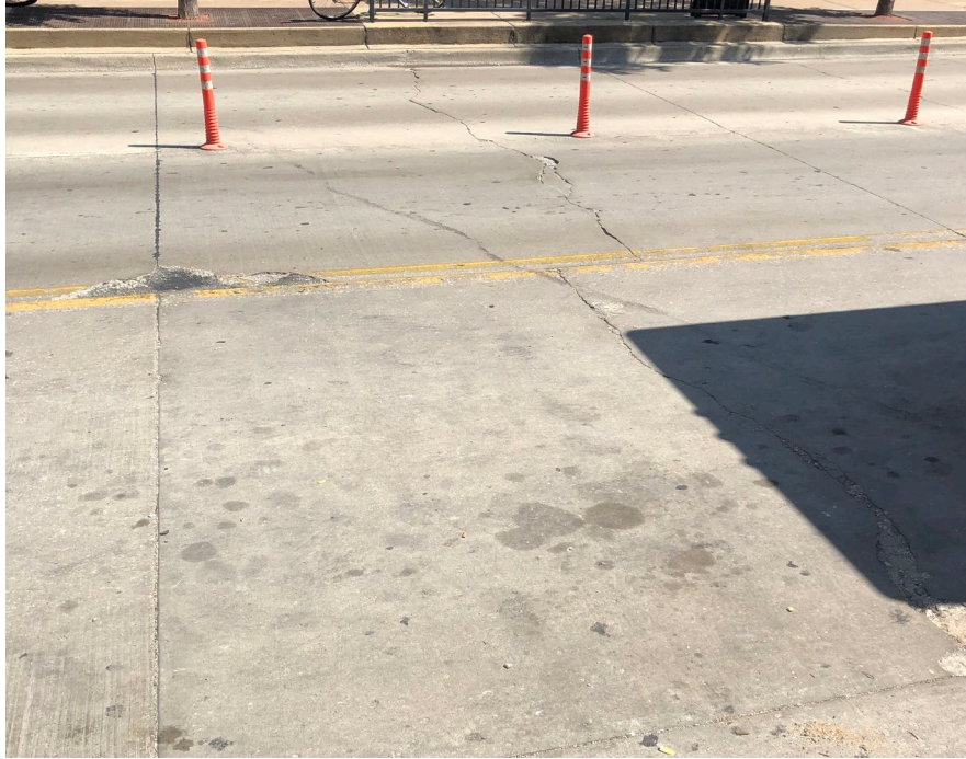
Figure 20. Photo. Transverse cracking on Green Street (Champaign, IL).
