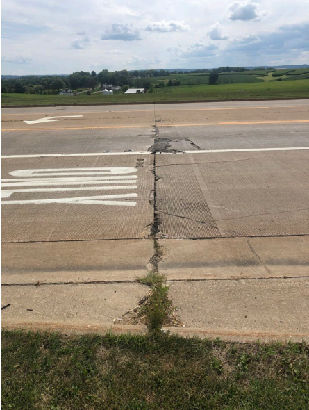
Figure 14. Photo. Transverse construction joint deterioration on US 20.
