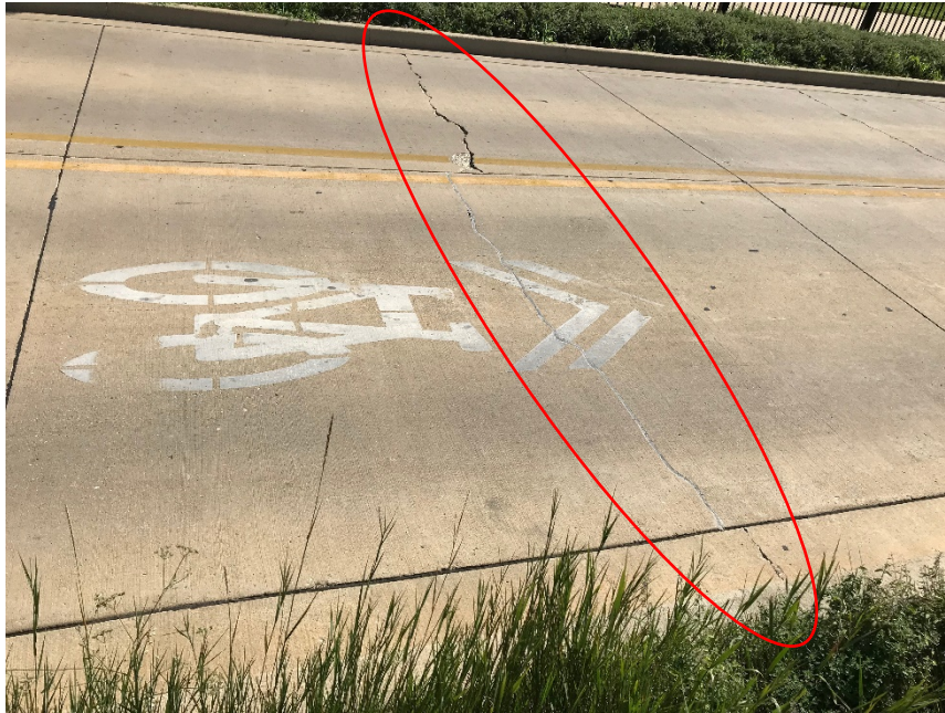
Figure S1. Photo. Urban concrete pavement section with a transverse crack.
