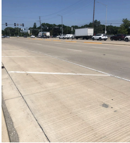
(A) IL 59 section constructed in 2002 (some cracking).
