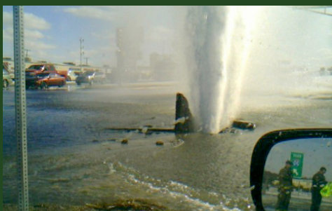
Drought and extreme heat causes roadway and utility rupture in Fort Worth, Texas. Photo credit: CBSDFW.com.
