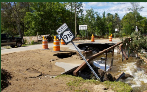
Culvert washout on New York State Route 9N during Tropical Storm Irene. Photo credit: Larry Master
