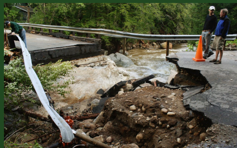
Culvert washout in the Lake Champlain Basin during Tropical Storm Irene. Photo credit: Naj Wikoff
