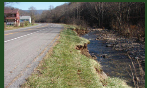
Example of roadside erosion in Maryland. Photo credit: SHA.
