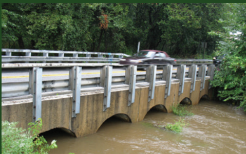
Large culvert over Sawmill Creek in Anne Arundel County that is vulnerable to heavy precipitation. Photo credit: MD Department of Environment.
