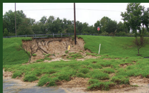
Roadway segment failure from a severe weather event. Photo credit: SHA.
