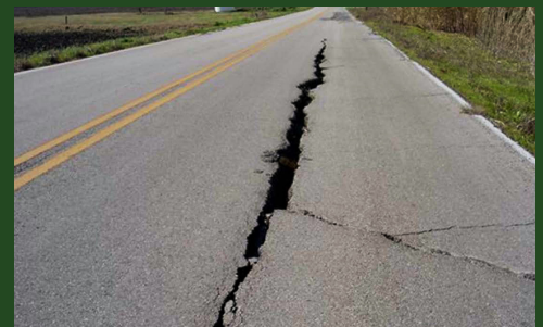
Severe pavement crack on Hamann Lane in Travis County during a drought in 2005. Photo credit: Scott Lambert, PE, Pavement Management Engineer, Travis County.
