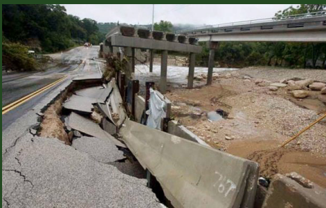
Damage to RM 2222 at the Bull Creek crossing due to overnight flooding September 7-8, 2010 (Tropical Storm Hermine). Photo credit: Austin American-Statesman.
