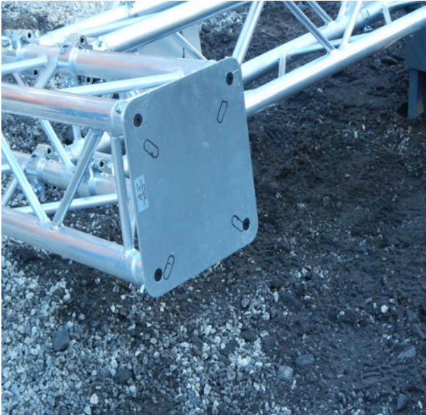
Figure 3. Bases Marked and Holes Drilled to Maintain the Exact Distance from the Rail
